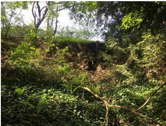
Stormwater outfall from the upper playing fields.
