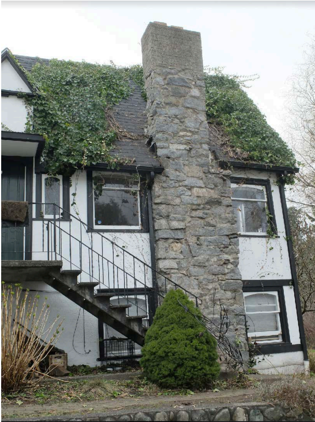
1st Street granite & concrete brick top chimney exposed after vine removal in early 2021.
