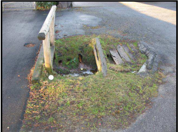
Existing unsightly gap b/n two culverts
