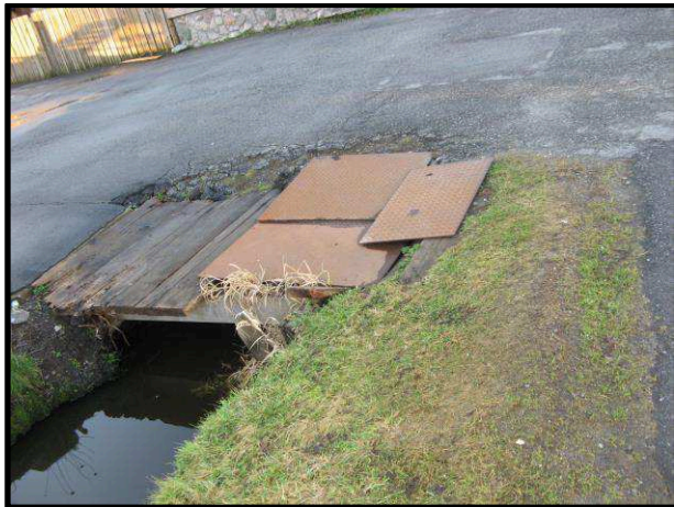
Existing unsafe pedestrian crossing ditch cover
