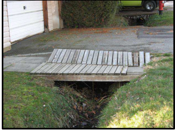
Existing unsafe pedestrian crossing ditch cover
