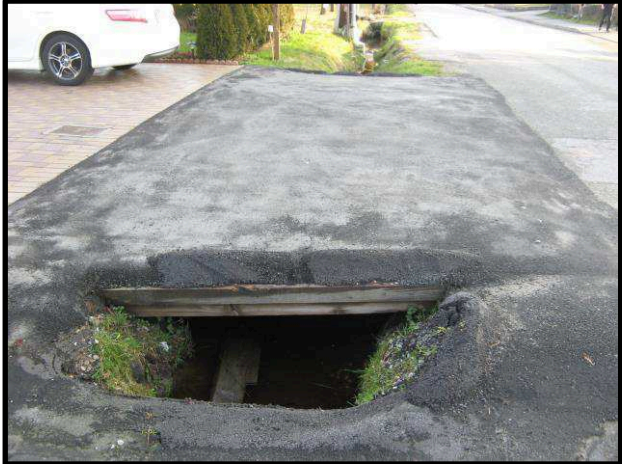
Existing unauthorized D/W culvert extensions
