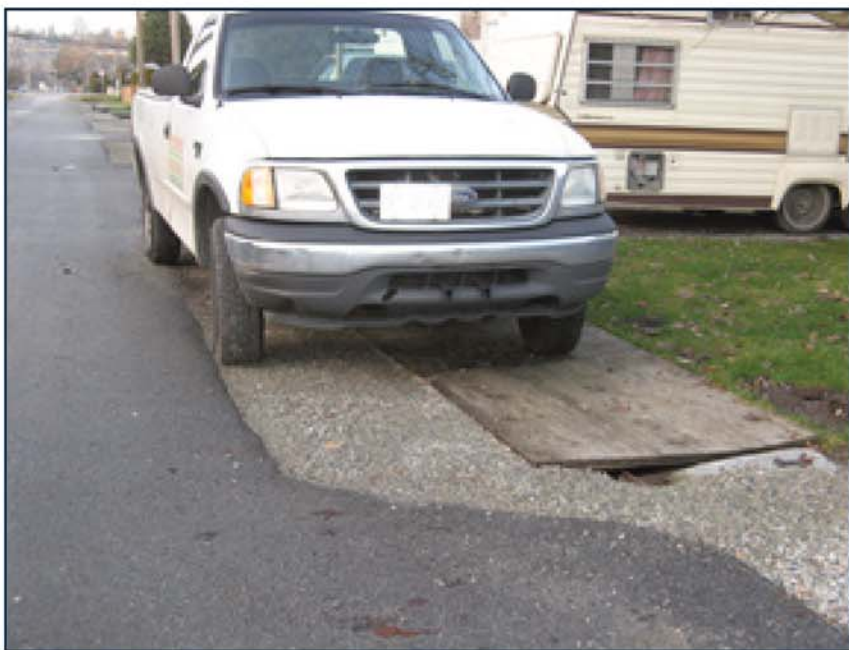
Existing hazardous plywood ditch cover.
