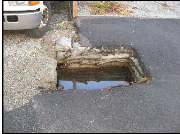
Existing unsafe gap b/n two D/W culverts
