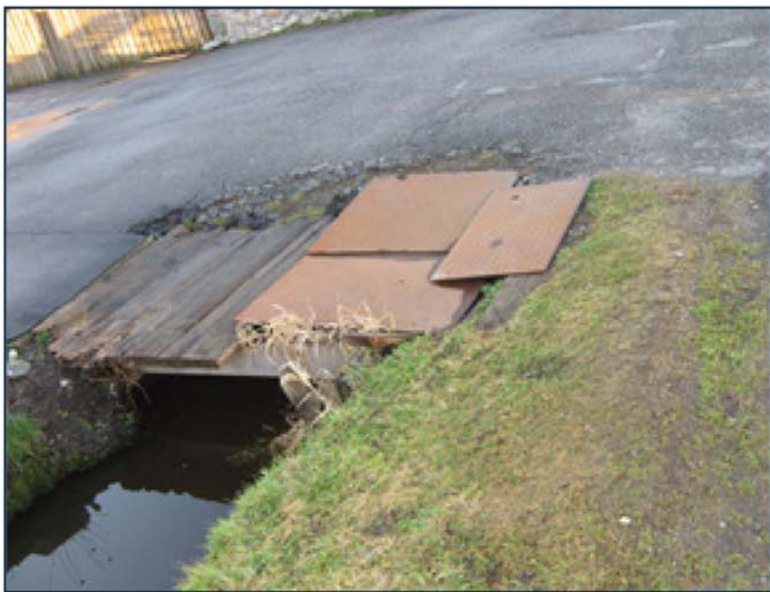
Existing non-standard rotten wood retaining wall.
