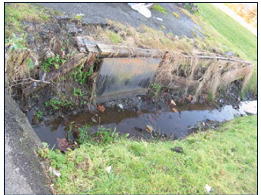
Existing hazardous pedestrian ditch crossing.
