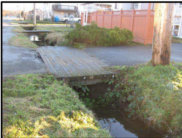
Existing non-standard wood cribbing
