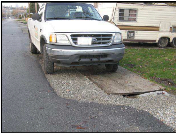
Existing unsafe plywood ditch cover
