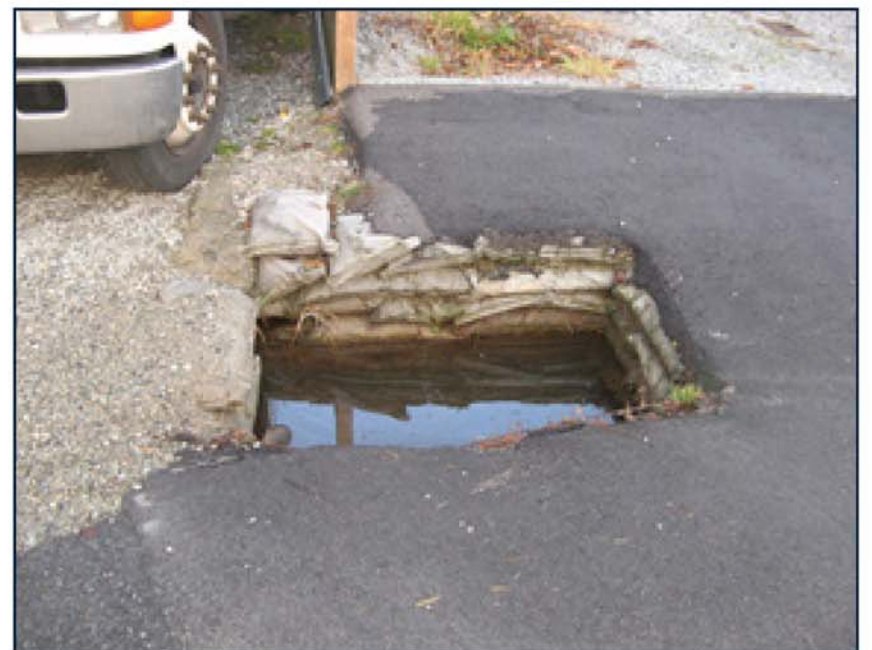
Existing hazardous gap between two driveway culverts.
