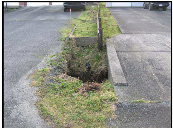
Unsafe gap b/n two immediate D/W crossings
