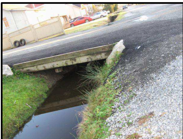
Existing unauthorized D/W crossing extension
