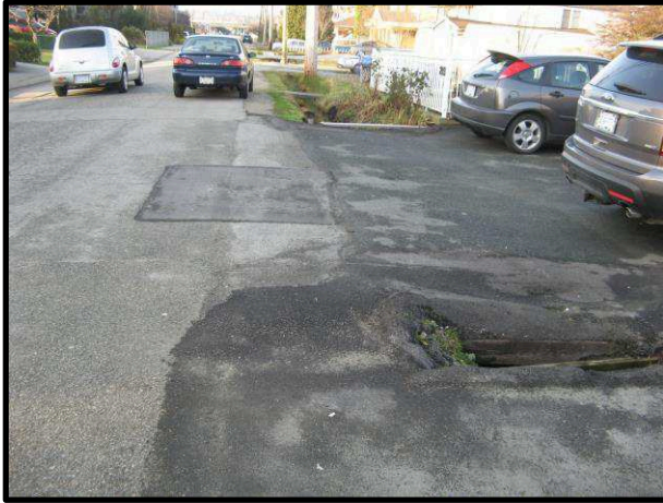
Existing unsafe gap between two driveway culverts
