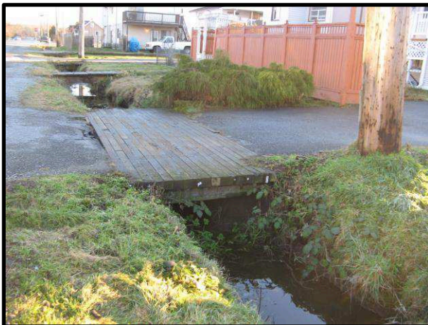
Existing non-standard wood cribbing
