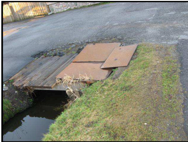
Existing unsafe pedestrian crossing ditch cover
