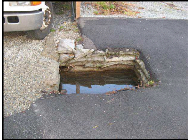
Existing unsafe gap b/n two D/W culverts
