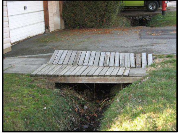
Existing unsafe pedestrian crossing ditch cover
