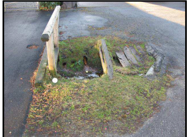
Existing unsightly gap b/n two culverts
