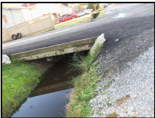
Existing unauthorized D/W crossing extension
