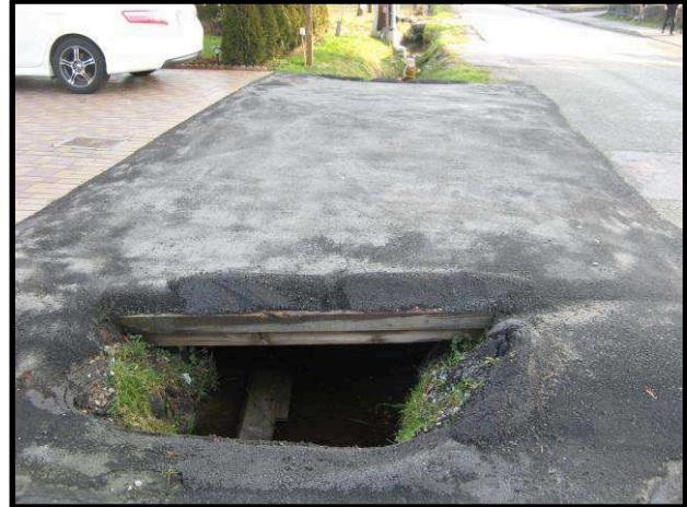
Existing unauthorized D/W culvert extensions
