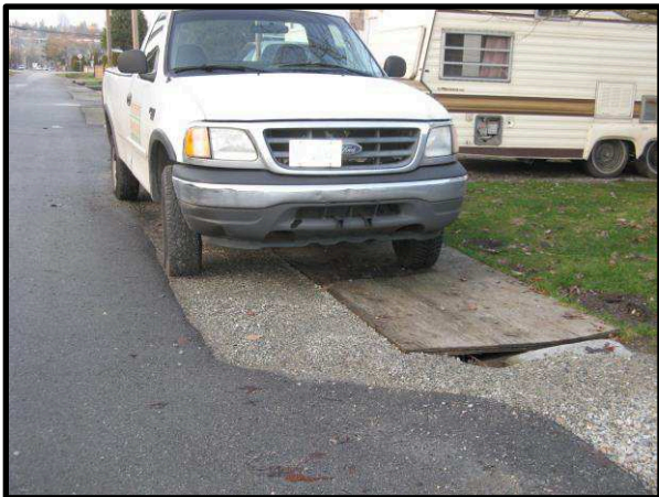
Existing unsafe plywood ditch cover
