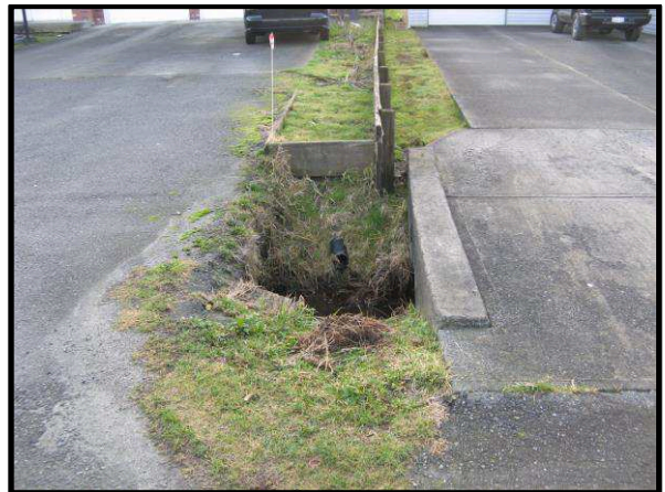
Unsafe gap b/n two immediate D/W crossings
