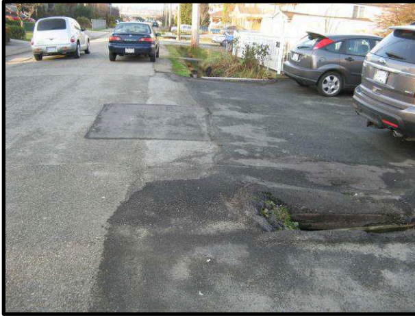
Existing unsafe gap between two driveway culverts
