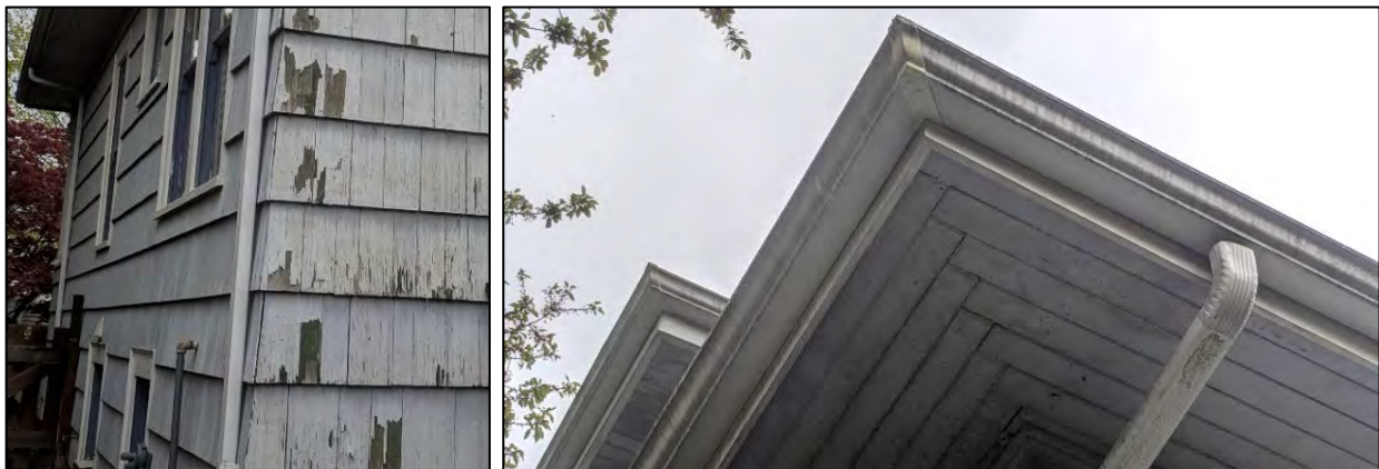
Figs. 29 and 30: Fig. 29 (left) shows the southwestern corner of Calbicks House at 208 Fifth Avenue, 2019, illustrating one area of the wood siding in need of repair; Fig. 30 (right) shows the southeastern corner soffit and fascia boards in need of minor maintenance. (Sources: Cummer)
