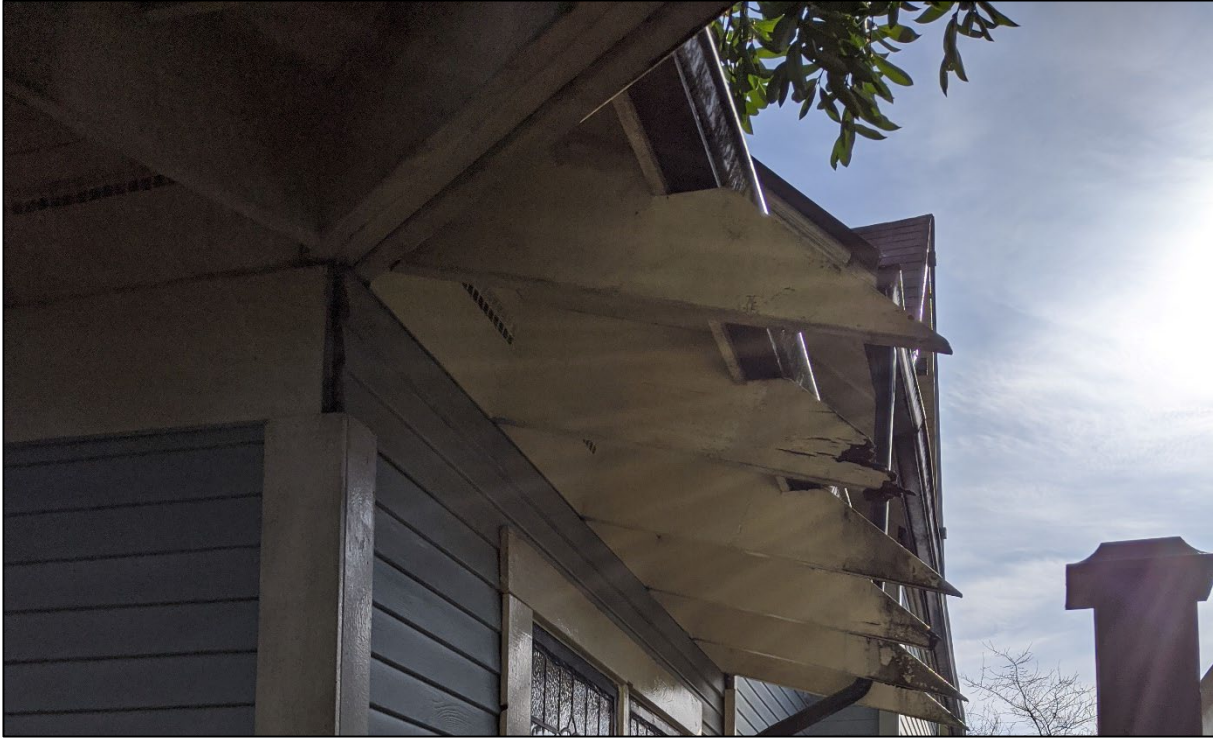
Fig. 12: Western side of Adams House at 515 St George Street, showing the dirty rafter tails, in need of cleaning and repainting, as well as ones in need of repair. (Source: Cummer)
