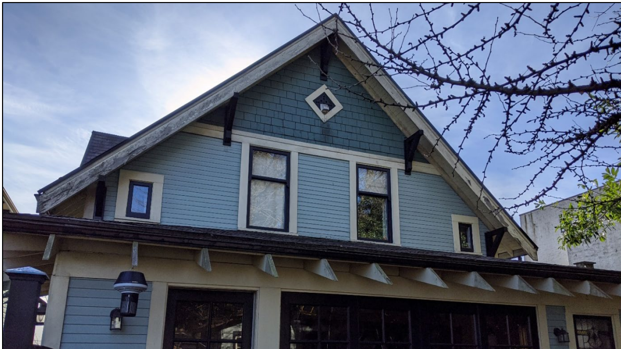
Fig. 11: Back gable of Adams House at 515 St George Street, showing the dirty rafter tails and soffits as well as the peeling fascia boards, in need of repainting. (Source: Cummer)
