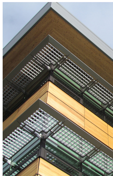
Exterior solar shading designed to shade during the summer and allow light in during the winter.
