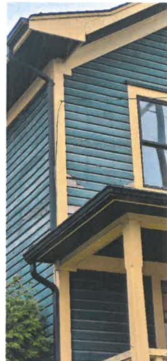
Front Elevation showing loss of paint.
