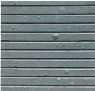
Side Elevation showing paint bubbling.
