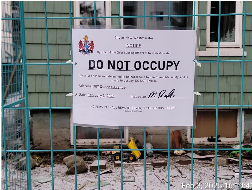
Picture 8: Do Not Occupy Order posted on front fence. Additional orders posted on rear and side yards.
