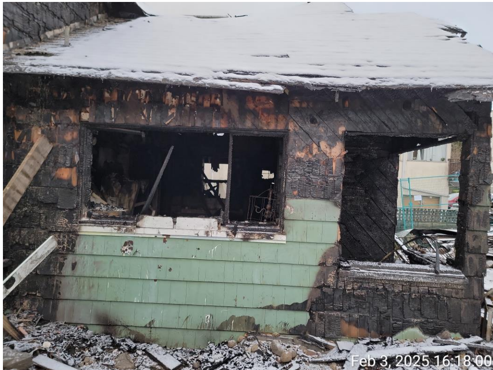
Picture 7: East side, rear portion of house. Significant damage to structure
