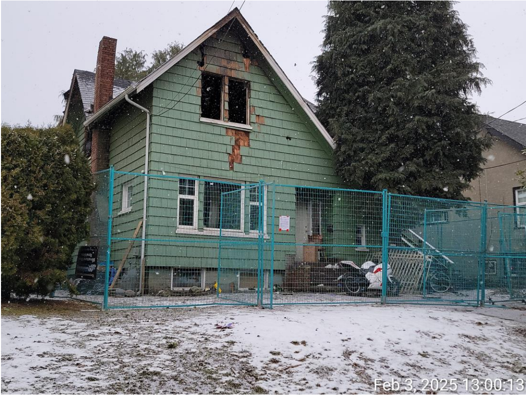
Picture 1: Front elevation of house. Windows on upper level blown out.
