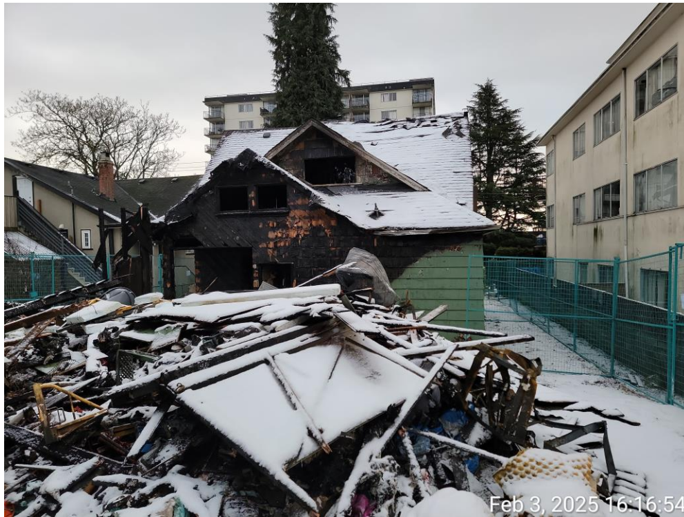
Picture 6: Rear of house, garage rubble in foreground. Note roof line sagging.
