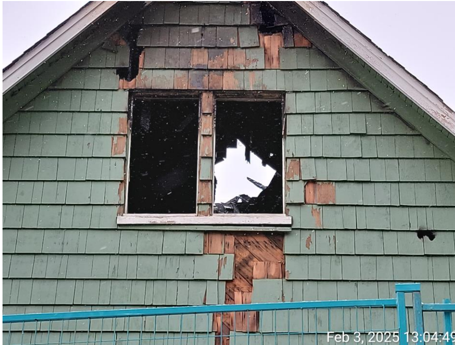
Picture 3: Collapsed roof. Current conditions do not comply with structural requirements of subsection 9.4 or Part 3 of the Building Code. Roof is not expected to support the minimum specified loads as required in subsection 9.4.2., for both snow and dead & live loads.
