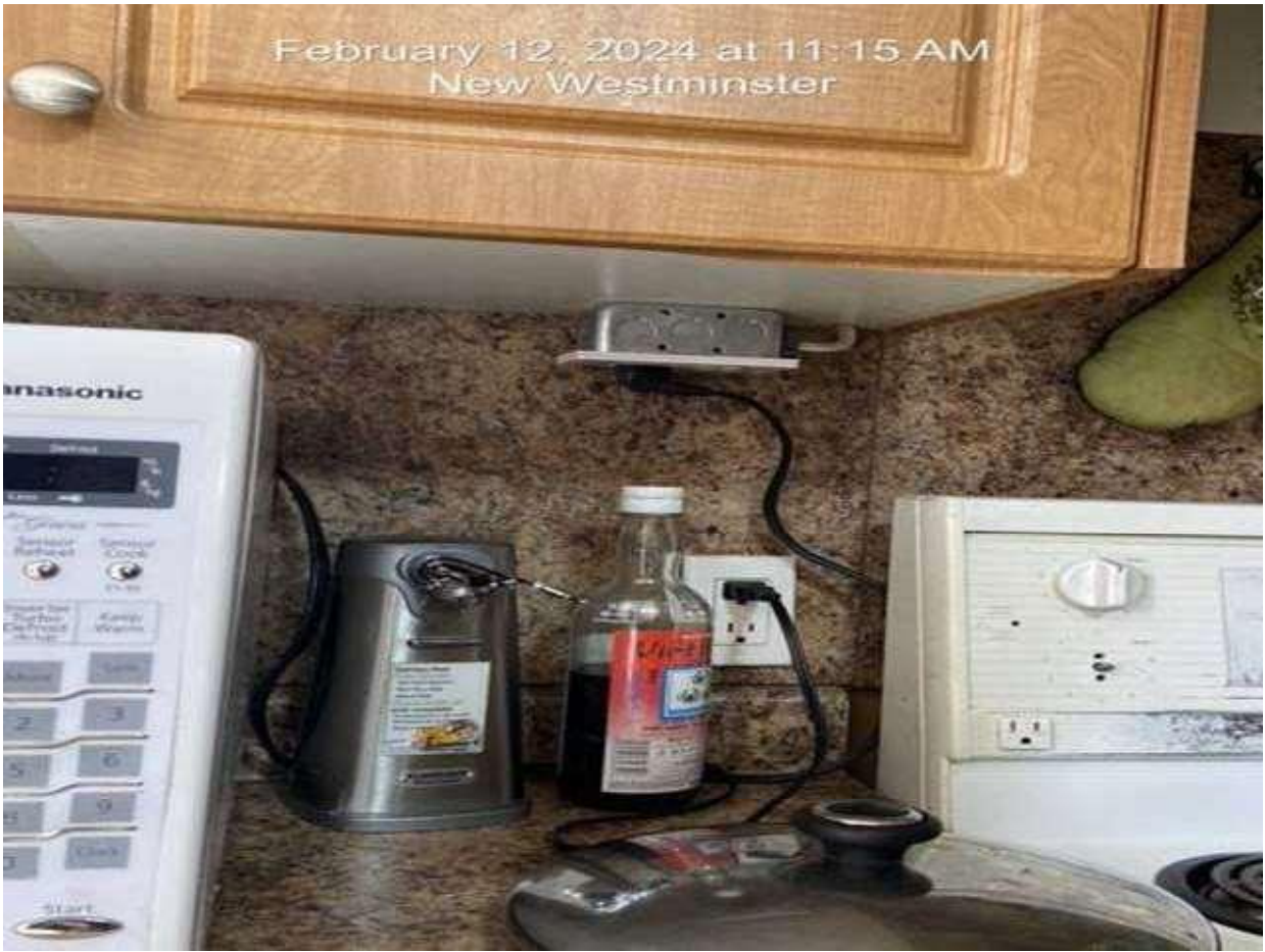
Pic 11 – ground level kitchen. Image of electrical wires running along walls.
