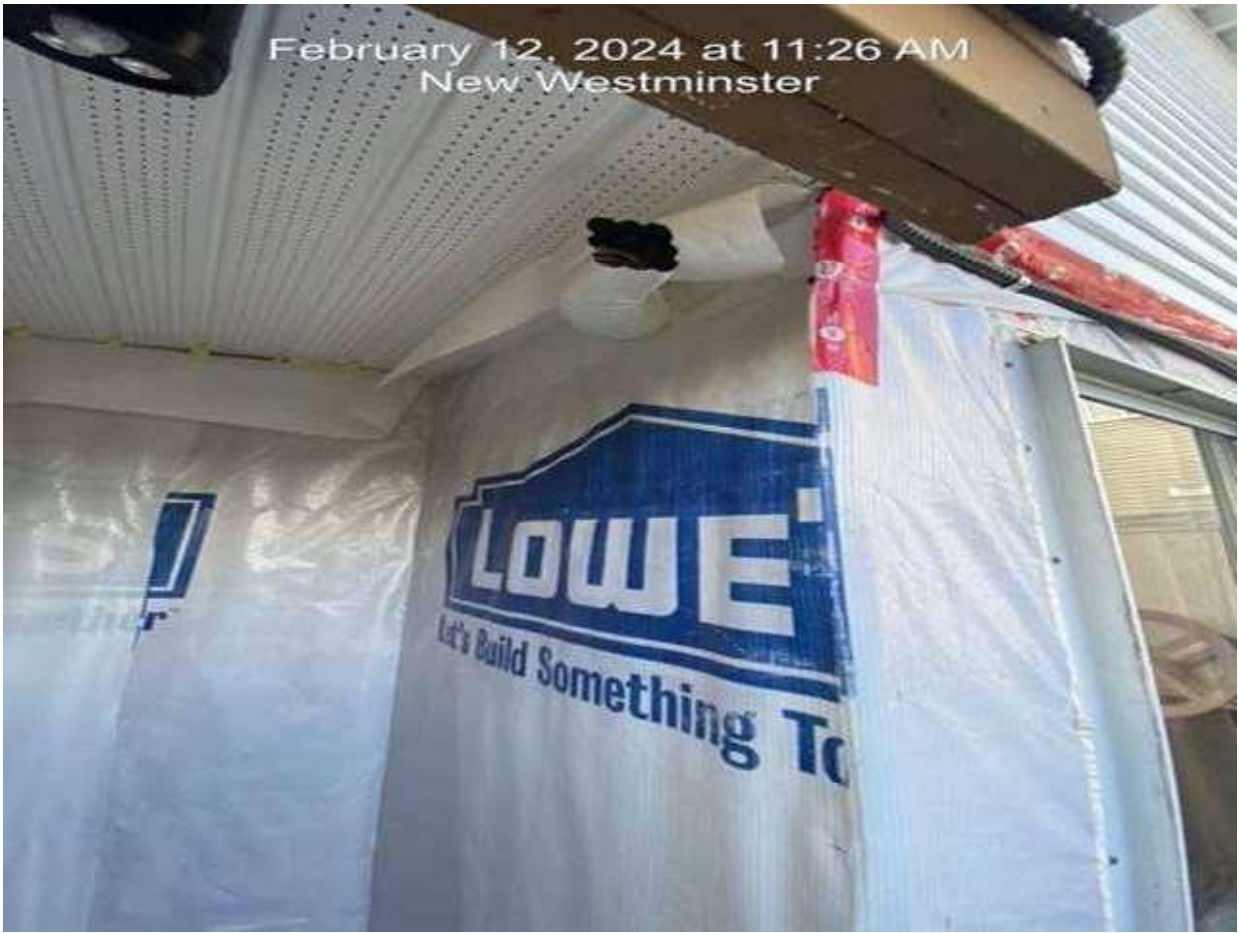
Pic 16 – ground level rear entry hallway. Electrical wiring taped along wall
