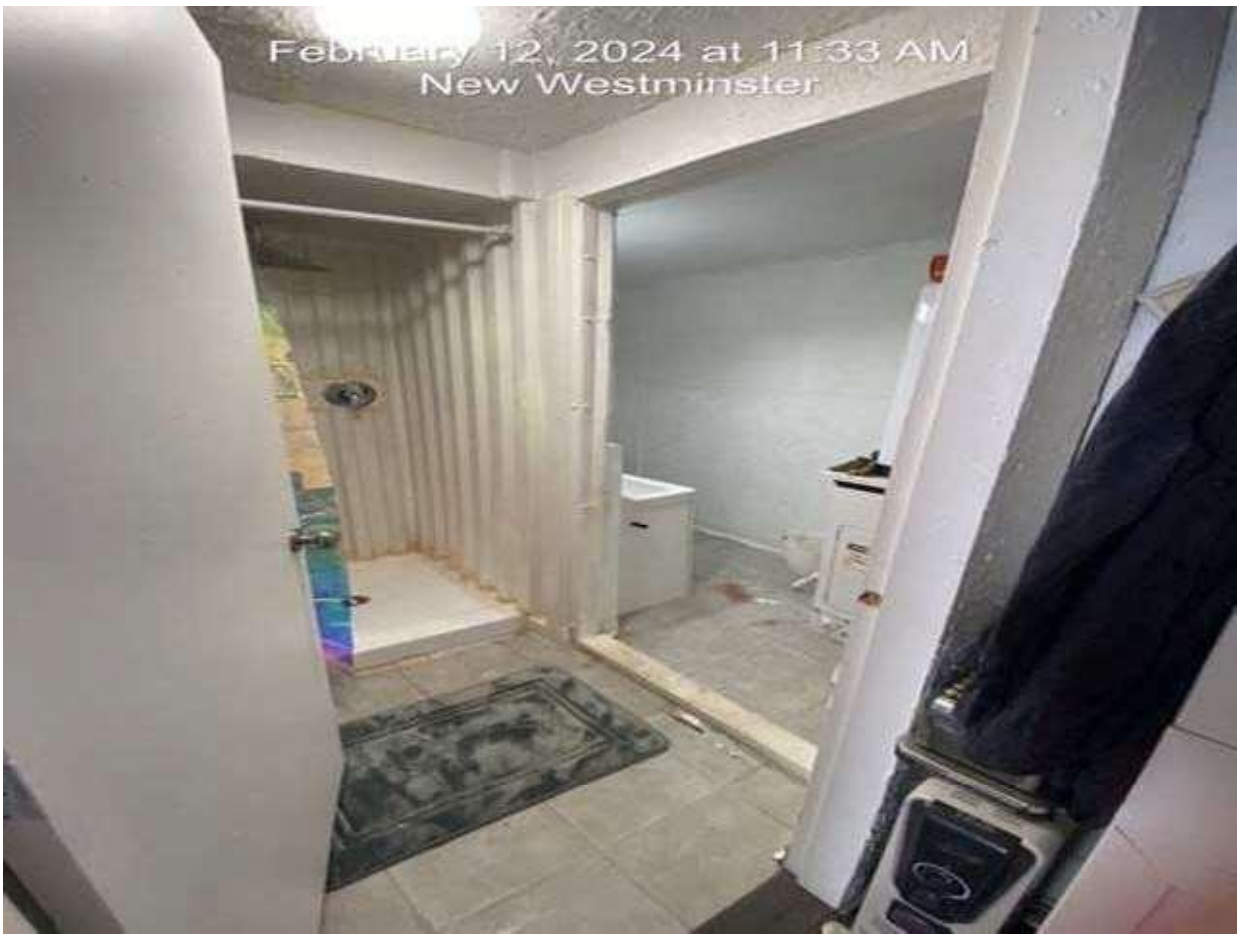
Pic 30 – second level north entry unit has a dryer in the bathroom
