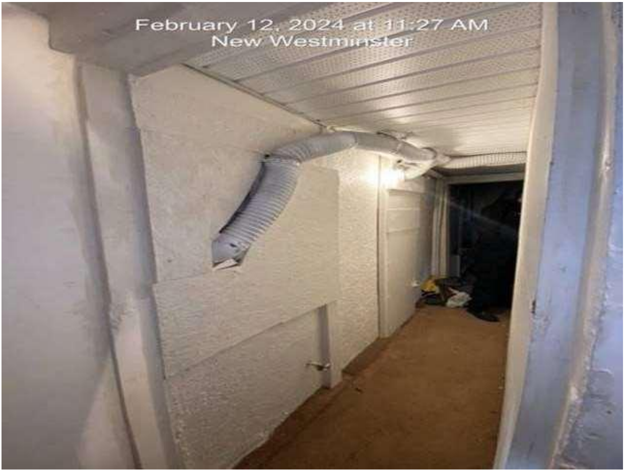
Pic 18 – ground level rear entry hallway, there is a power cord with misc lights plugged into it.
