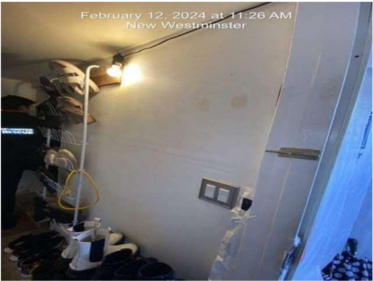
Pic 17 – ground level rear hallway to two units. Wall is an exterior wall on the left
