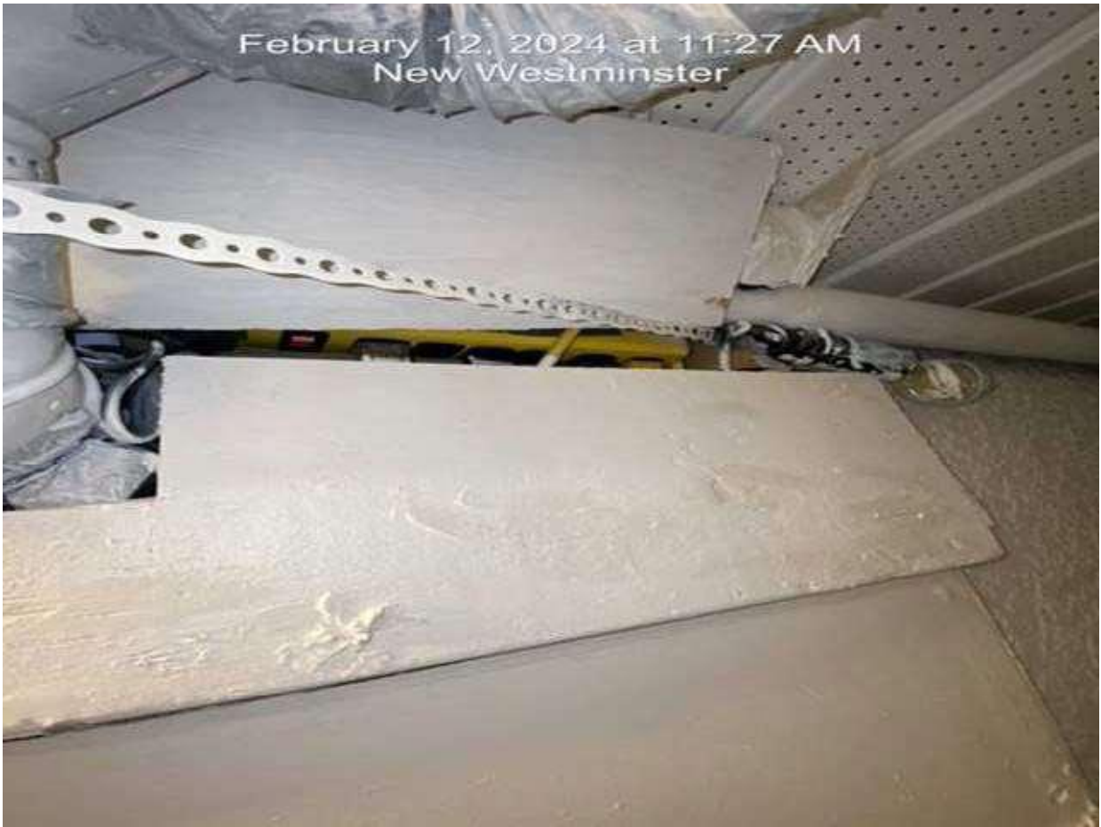
Pic 19 – ground level unit at rear. The ceiling is aluminum and there are exterior pipes running through the room
