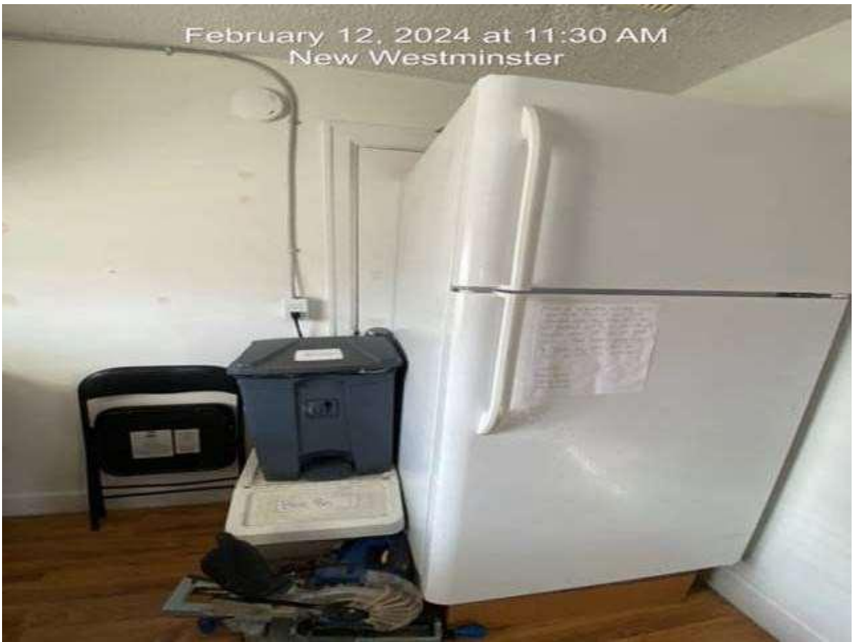
Pic 24 – ground level rear entry kitchen foundation is exposed and flooring uneven
