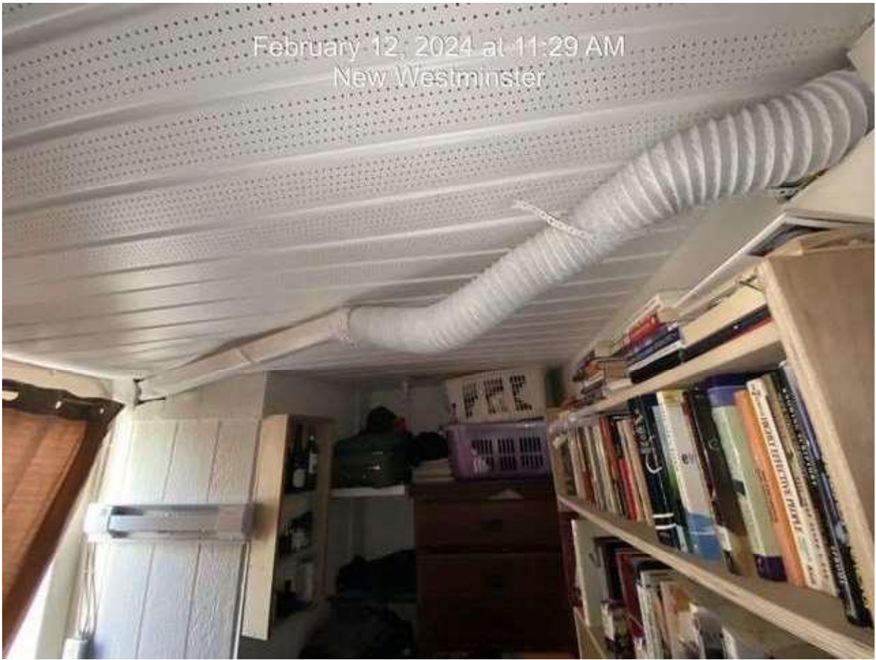
Pic 21 – ground level rear entry unit bedroom has aluminum ceiling and heater mid-wall
