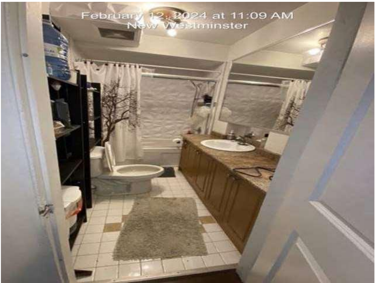
Pic 7 – second level. Wall to the left is hollow and taped together to create a wall.
