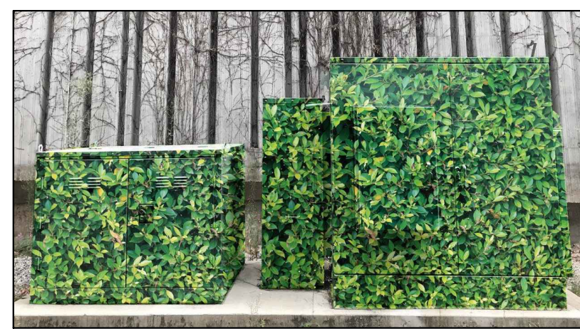
POSSIBLE SUBSTATION VINYL WRAP
