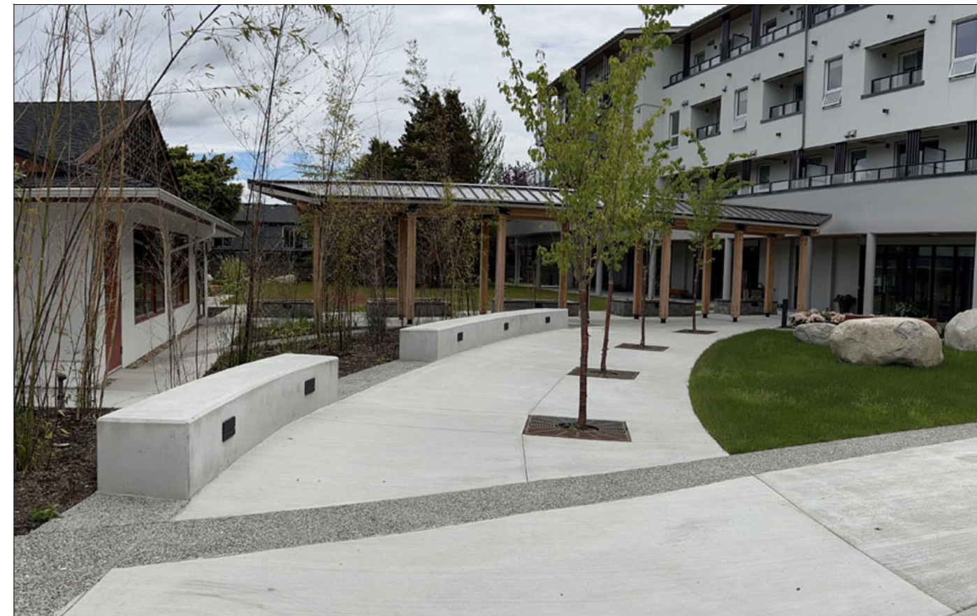
CONCRETE SEATWALL DESCRIPTION: CAST IN PLACE CONCRETE, SANDBLAST FINISH WITH WALL LIGHTING
