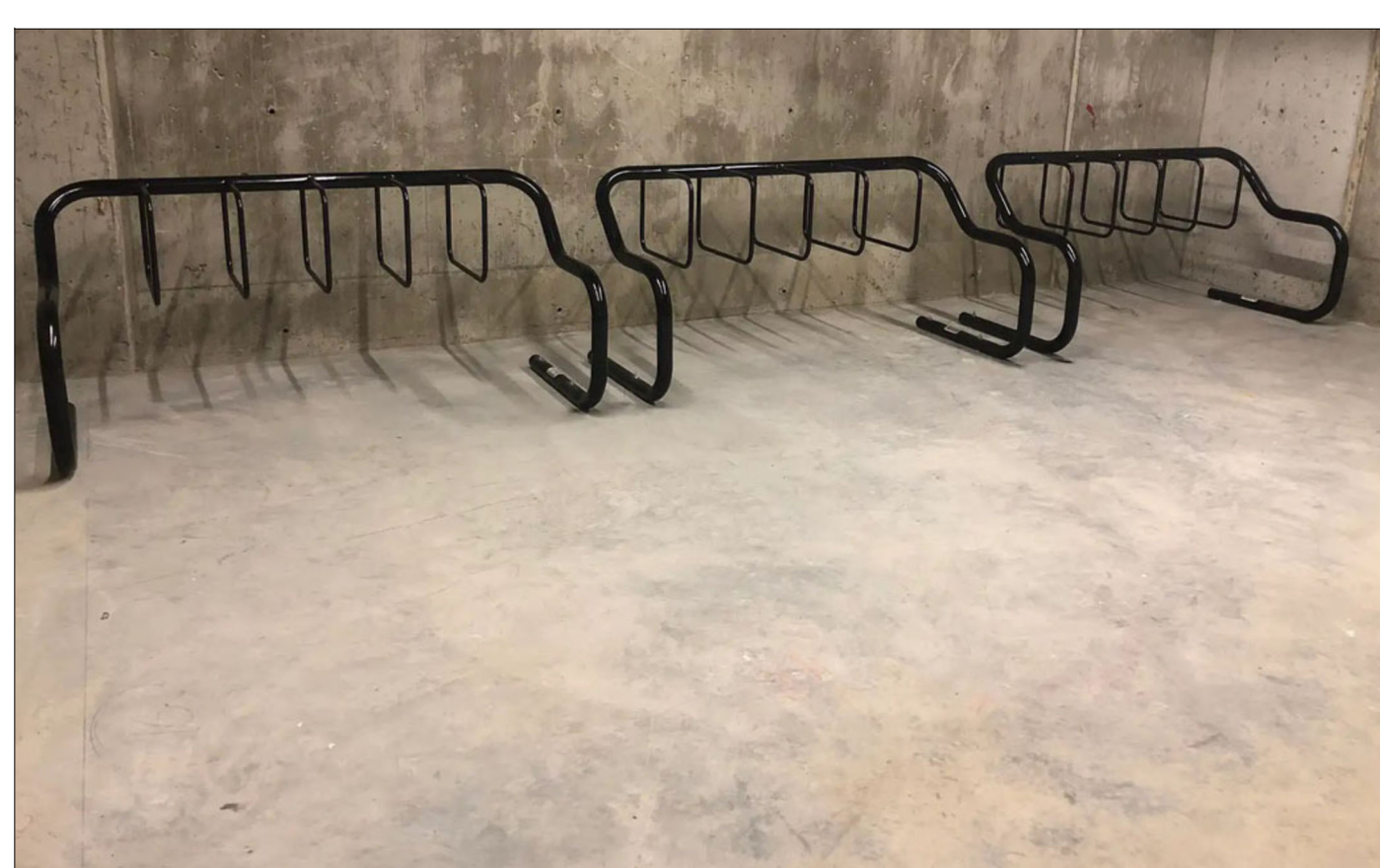
BICYCLE RACKS DESCRIPTION: METAL PIPE BIKE RACKS GALVANIZED OR POWDER COATED BLACK.
