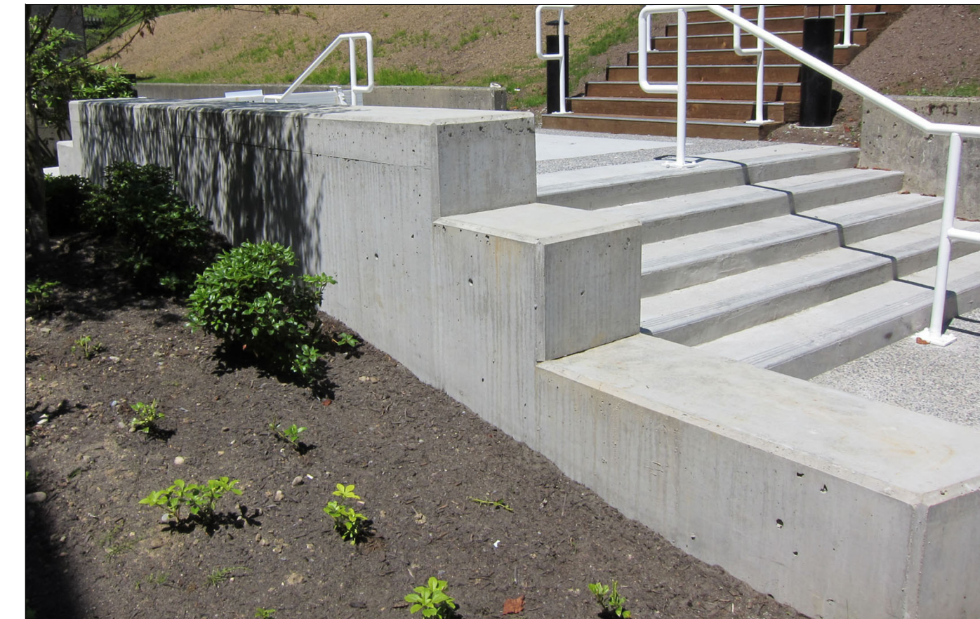
CONCRETE STAIR - SEATWALLS DESCRIPTION: CAST IN PLACE CONCRETE, SANDBLAST FINISH WITH EXPOSED AGGREGATE BANDS & HAND RAILS
