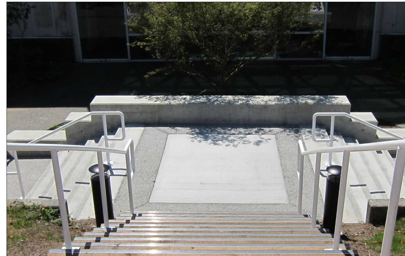
CONCRETE STAIR - LANDING DESCRIPTION: CAST IN PLACE CONCRETE, SANDBLAST FINISH WITH EXPOSED AGGREGATE BANDS & HAND RAILS
