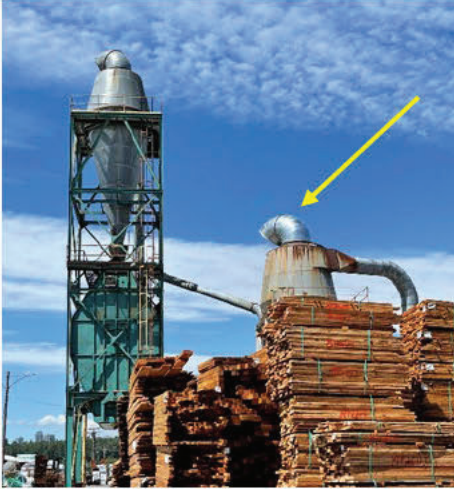
Cyclone #2 (ES-02, lower cyclone)
