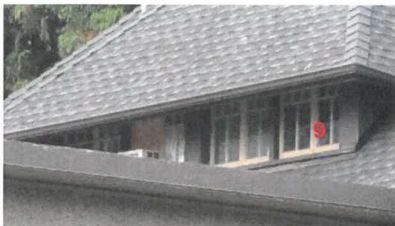
9 dormer double assembly windows. One sash is missing where an air conditioning unit was installed.
