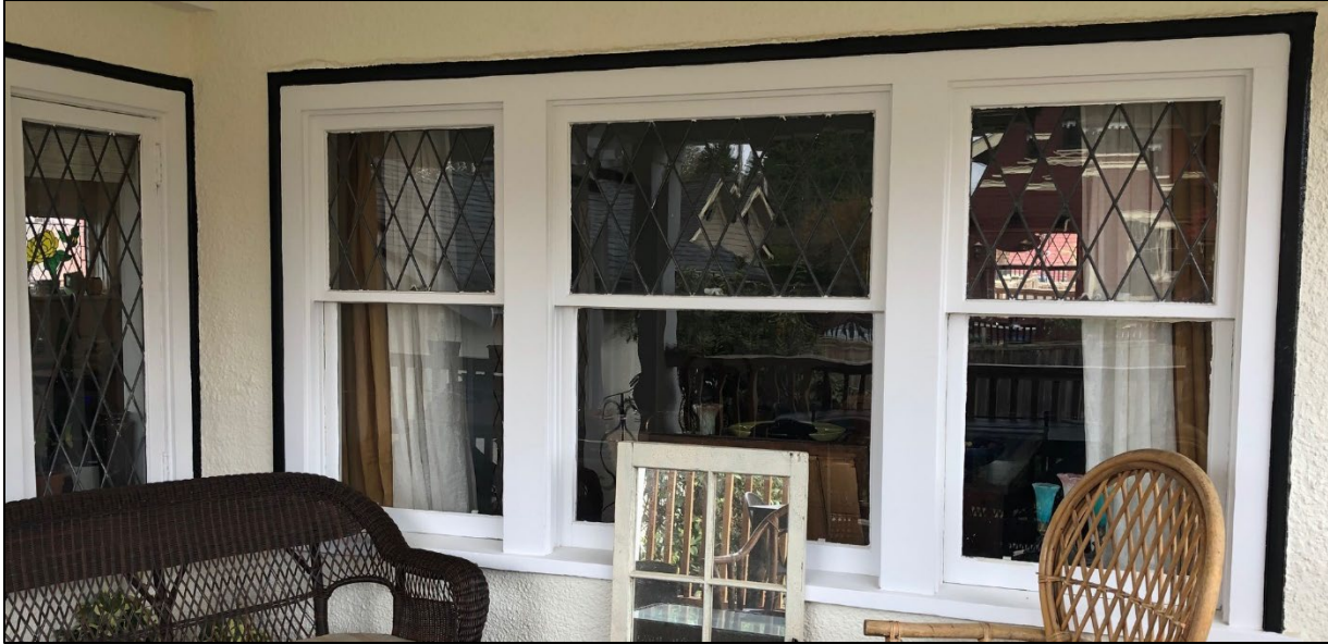
Fig. 22: The back deck of Edgar House at 323 Regina Street, 2020, illustrating the good condition of its original windows, with diamond patterned panes. (Source: Holisko)
