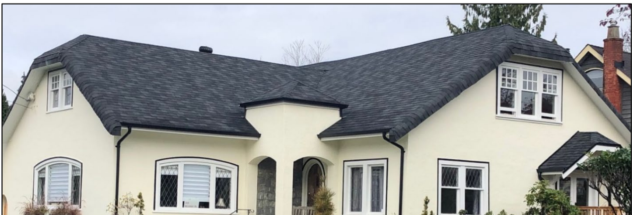
Fig. 19: Front view of Edgar House at 323 Regina Street, 2020, illustrating the good condition of its roof. (Source: Holisko)
