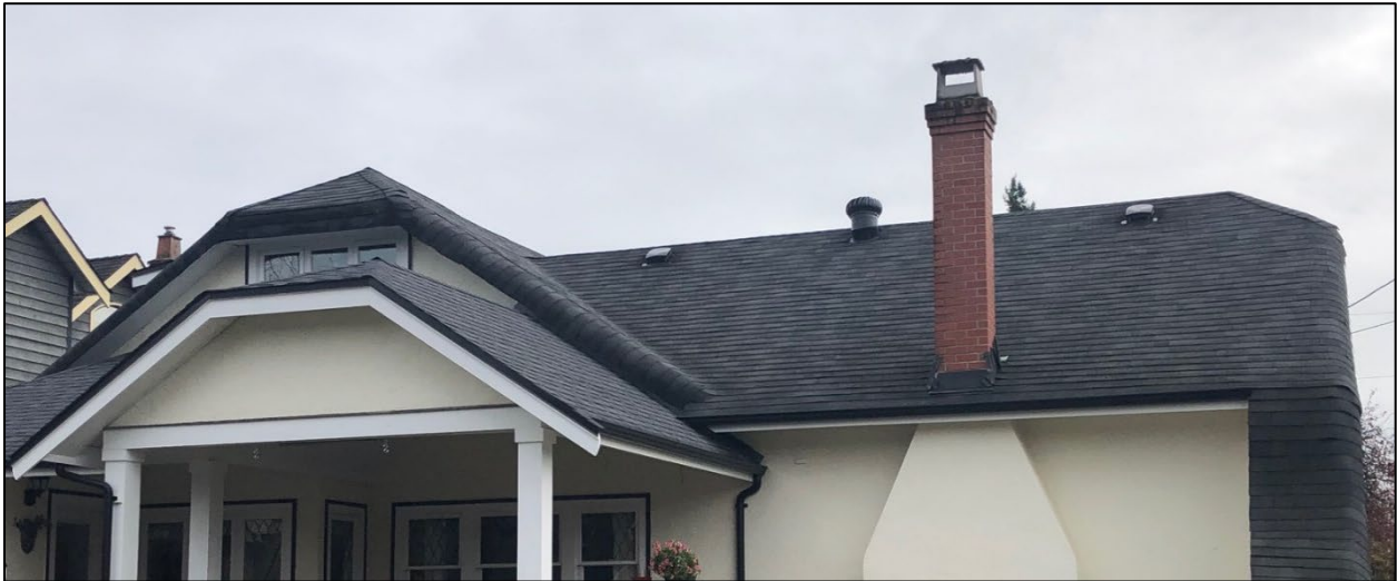
Fig. 20: Back view of Edgar House at 323 Regina Street, 2020, illustrating the good condition of its roof. (Source: Holisko)
