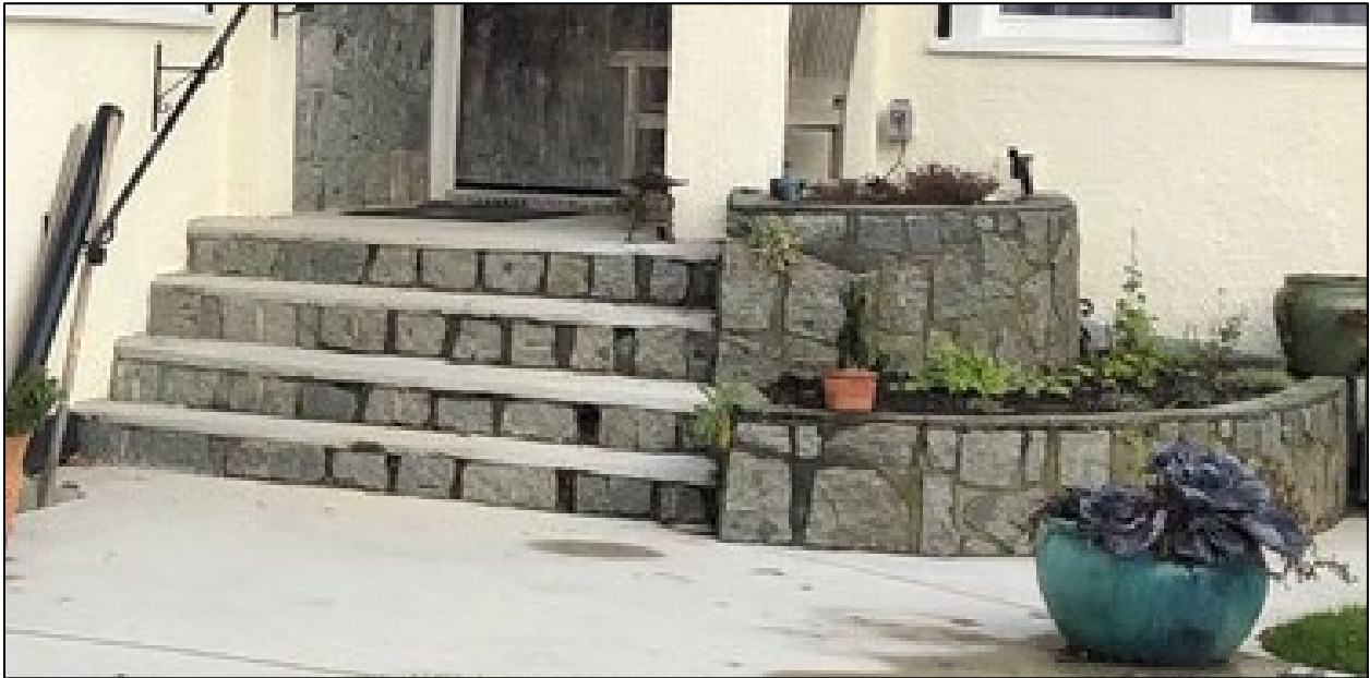
Fig. 18: Front stone steps and planter of Edgar House at 323 Regina Street, 2020, illustrating the minor maintenance concerns, such as moss growth and other plants growing between the stone slabs. (Source: Holisko)
