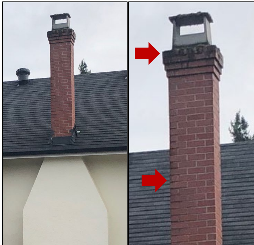
Figs. 21a and 21b: Fig. 21a (left) shows a detail shot of the Edgar House chimney, highlighting its largely good condition. Fig. 21b (right) shows a closer view of the chimney stack, showing some signs of deteriorating mortar and areas in need of cleaning (pinpointed by red arrows). (Sources: Holisko)
