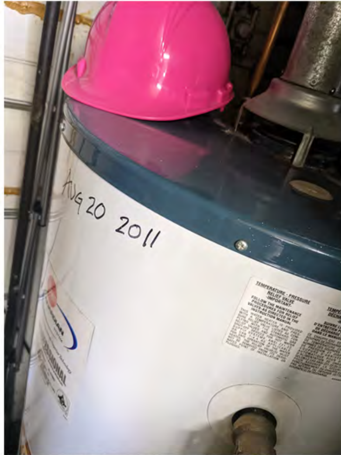
unit 349 - water heater installed in 2011.jpg
