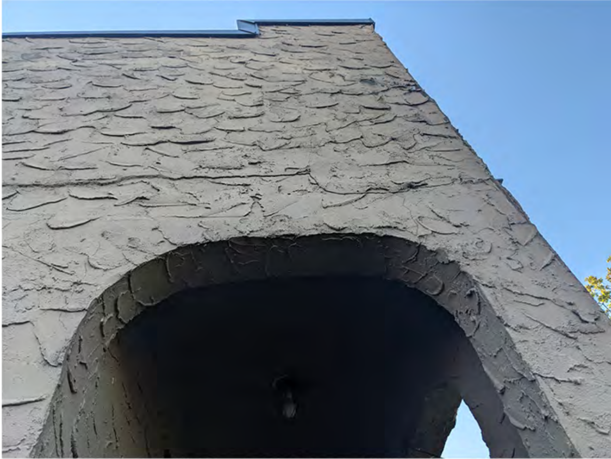
unit 349 - cracks in wall above east wall entryway.jpg
