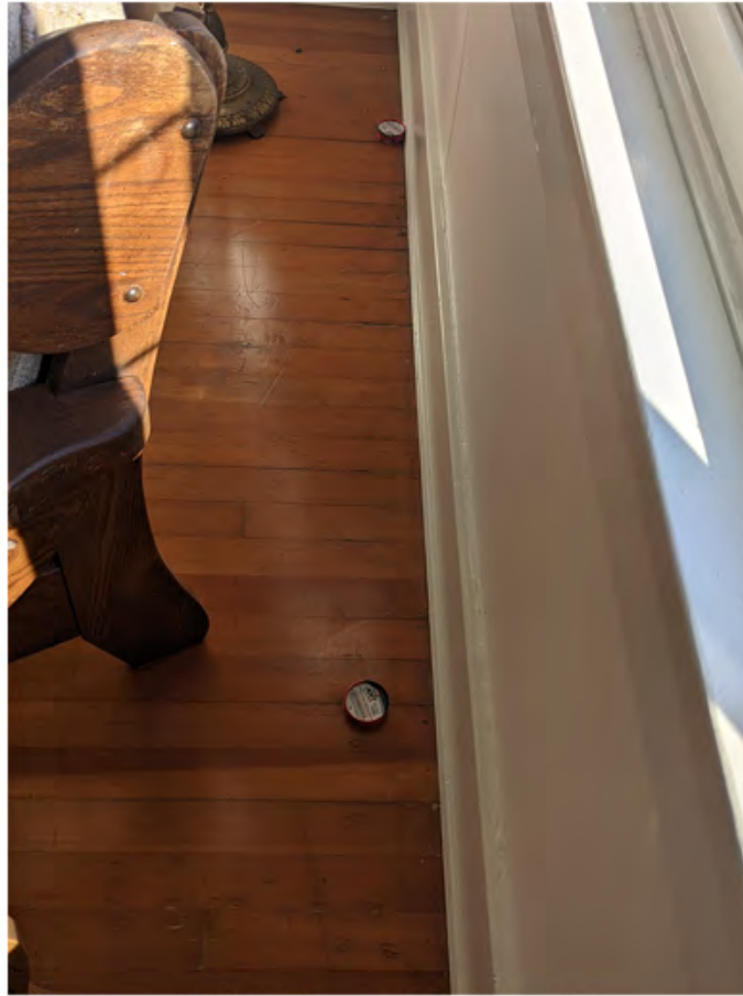
unit 349 - evidence of insect ingress.jpg
