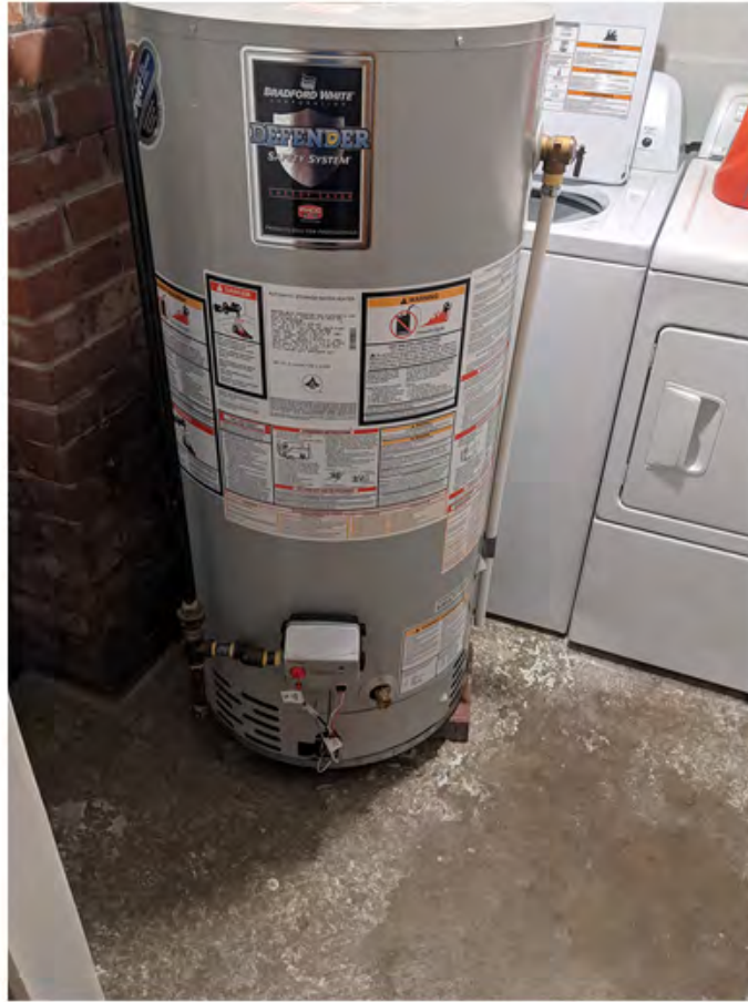
unit 351 - Bradford White HW heater MD 201210.jpg
