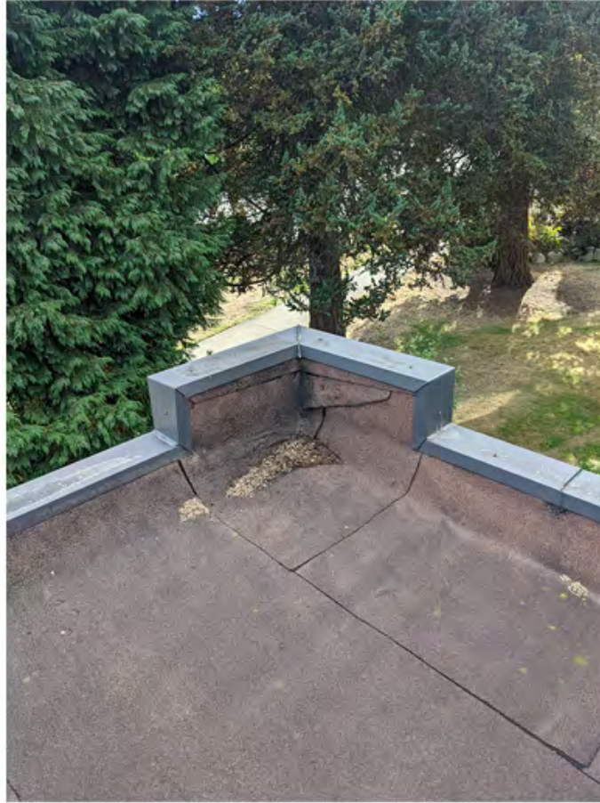
rolled asphalt seams degraded.jpg
