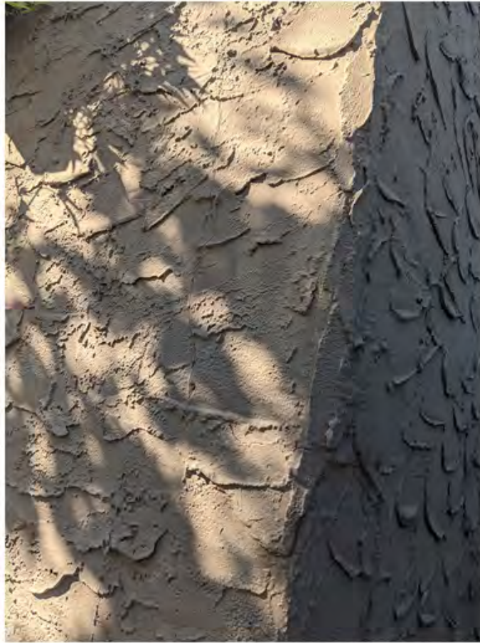
crack in stucco on south wall east side.jpg
