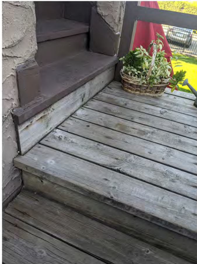
unit 349 - stairway wood near end-of-life.jpg
