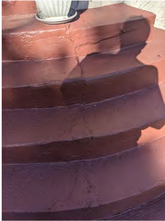
unit 349 - south entryway stairway cracks have increased in depth over the past 15 years.jpg
