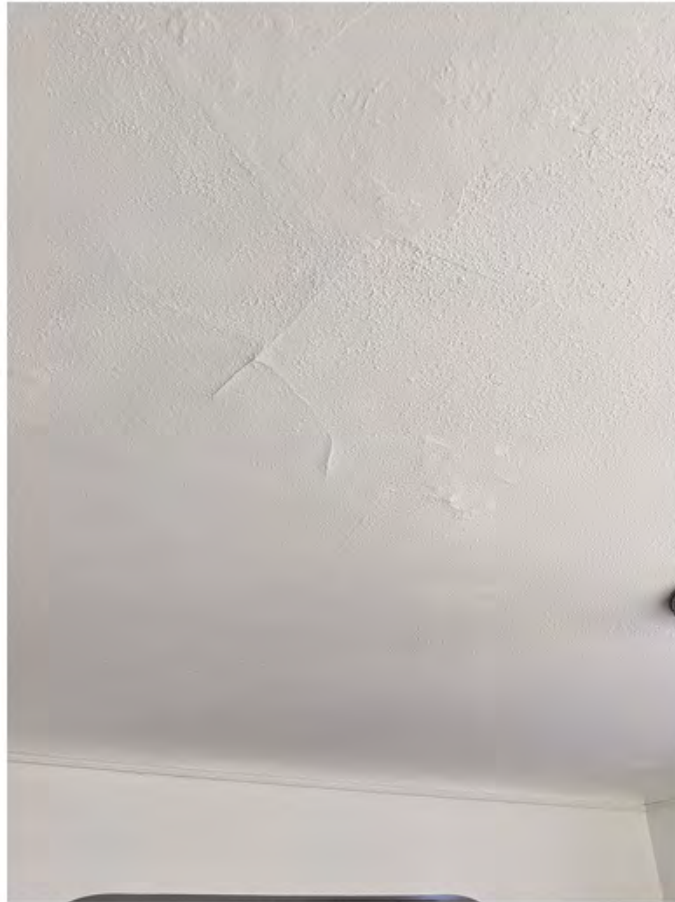
unit 349 - ceiling cracks.jpg
