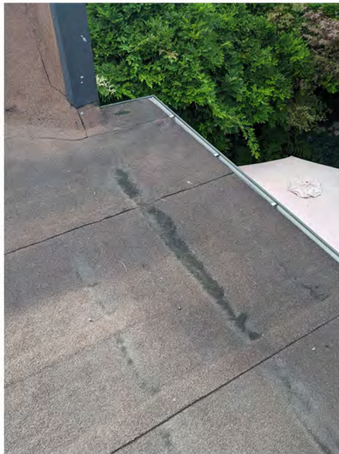
degraded rolled asphalt due to ice damming.jpg
