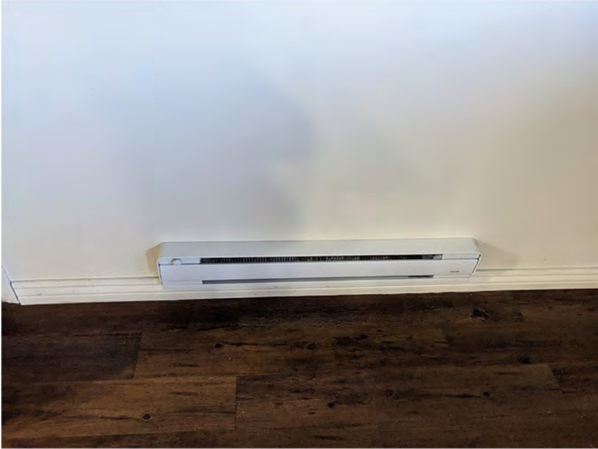
unit 349 - lower level baseboard heater.jpg
