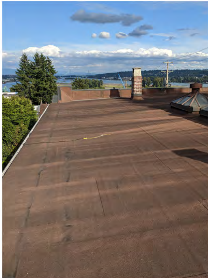
rolled asphalt no longer laying flat.jpg
