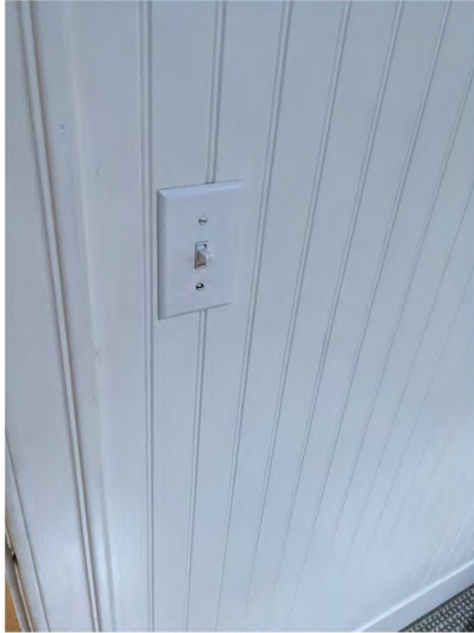
unit 351 - light switch likely requires replacement.jpg
