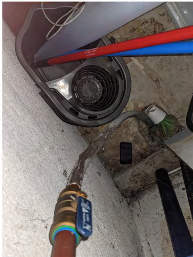
unit 349 - water supply to Subject Building with no meter and potential lead piping.jpg
