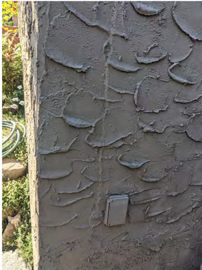
crack in stucco on east wall south side.jpg
