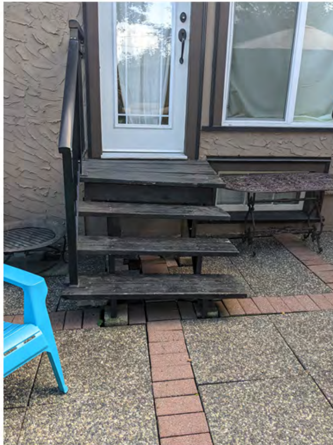
unit 351 - settlement in north entryway stairway.jpg
