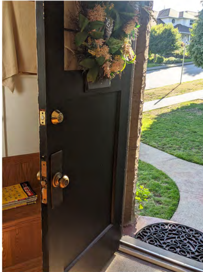
unit 349 - south doorway needs to be replaced due to settlement and faulty hardware.jpg
