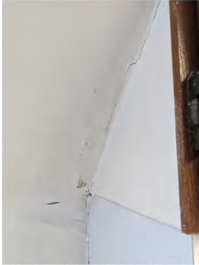
unit 349 - evidence of moisture ingress above stove in lower level likely from building envelope failure.jpg
