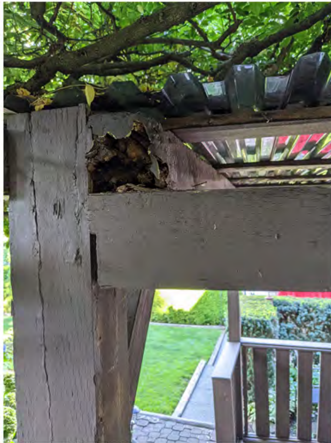
unit 349 - pergola with evidence of extensive rot.jpg
