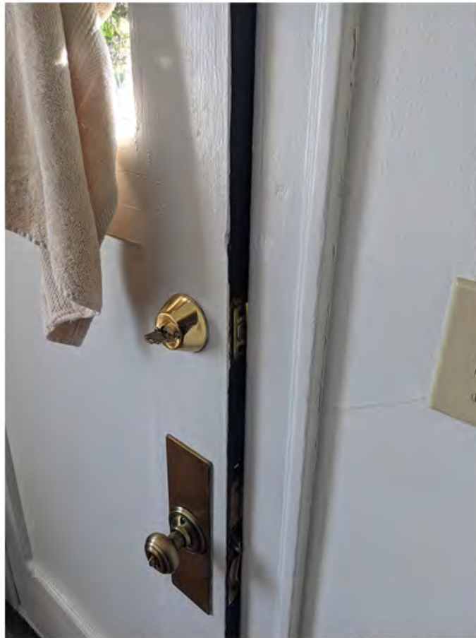
unit 349 - south doorway binding on open and closure.jpg
