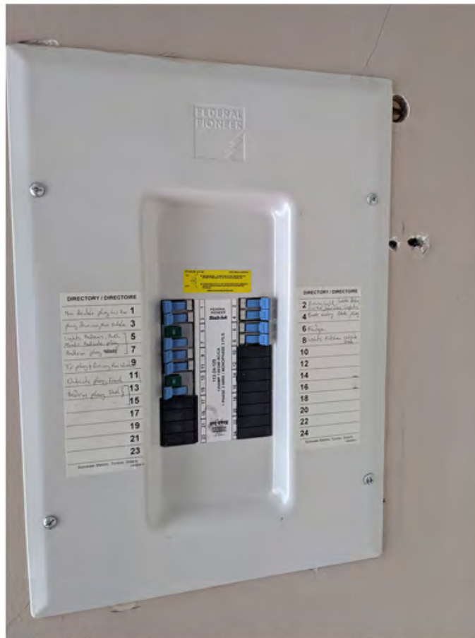
unit 351 - electrical panel west of WC on main level.jpg
