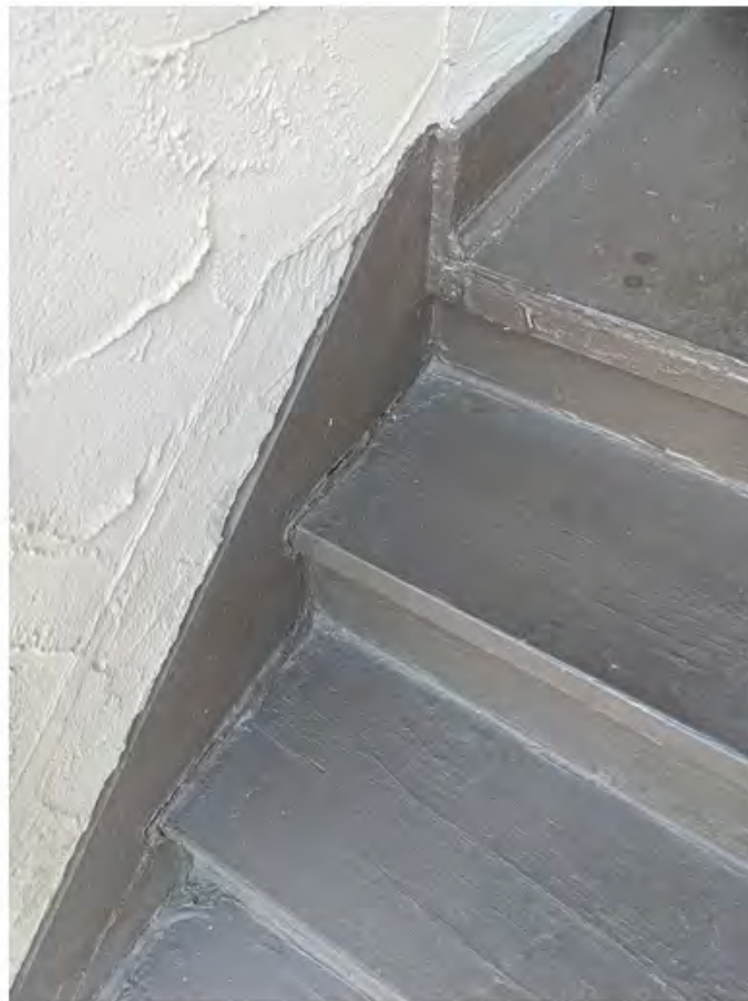
unit 349 - cracks in stairwell up to south egress doorway.jpg
