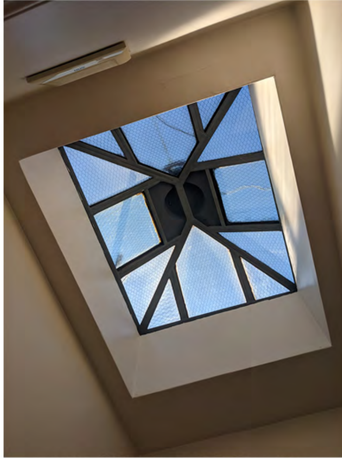
unit 349 - sky light in upper level WC with cracks.jpg
