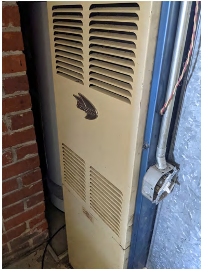
unit 349 - mid efficiency furnace likely at end-of-life with no replacement heat exchanger possible.jpg
