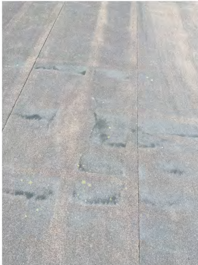
roof surface with degraded granular material.jpg
