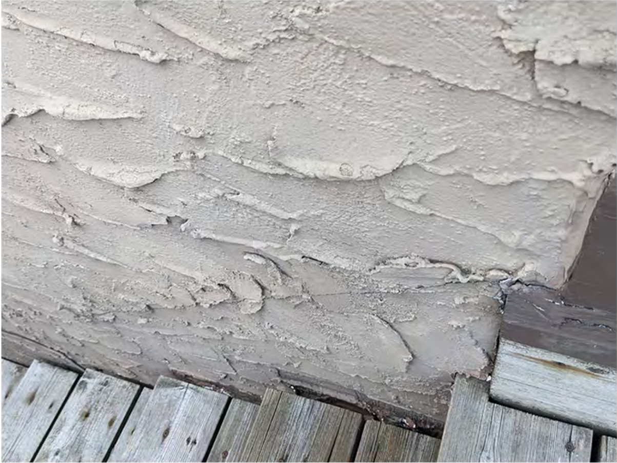
unit 349 - outer east wall stairway with evidence of settlement cracks.jpg
