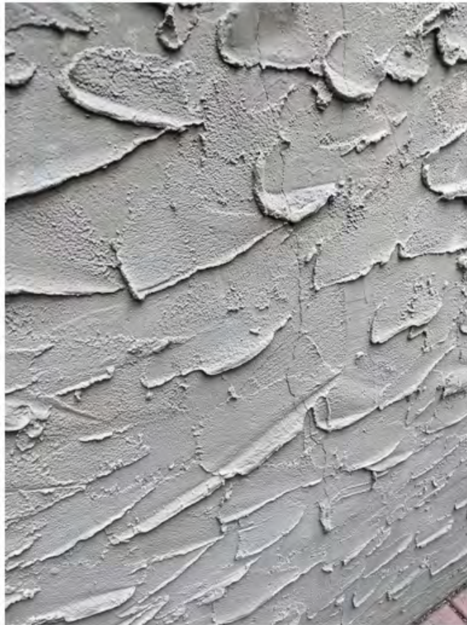
crack in stucco on west wall central area.jpg
