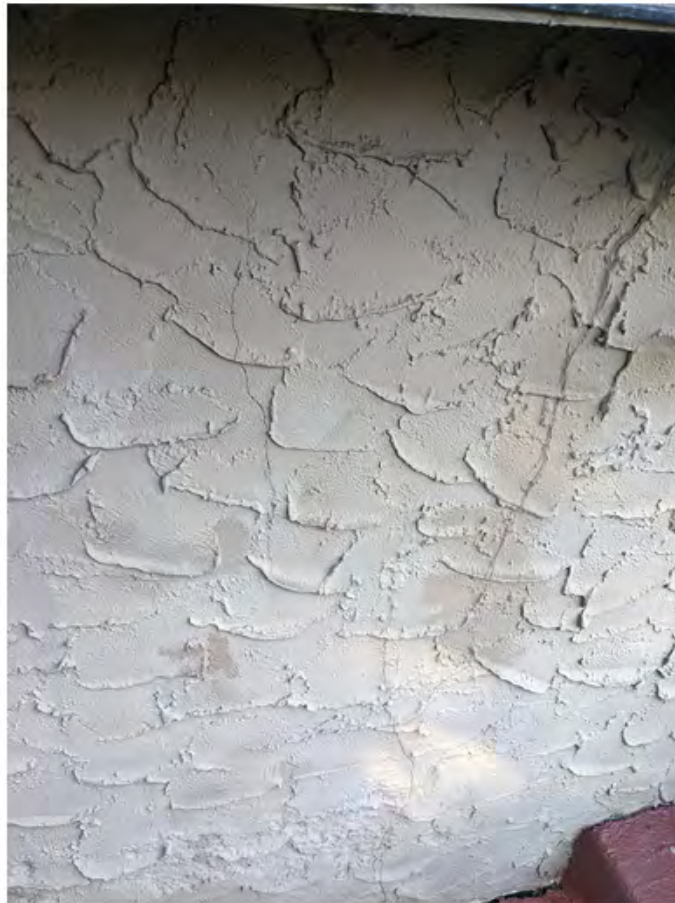
unit 349 - cracks in stucco on south wall justt west of entryway door.jpg
