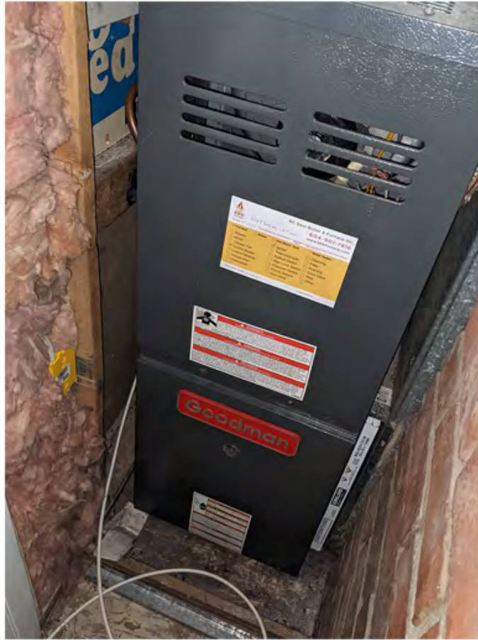
unit 351 - likely high efficiency goodman furnace.jpg
