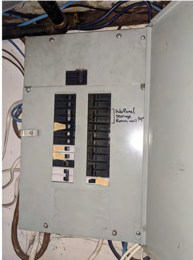
unit 349 - 100Amp electrical panel in lower level on east wall - south side.jpg
