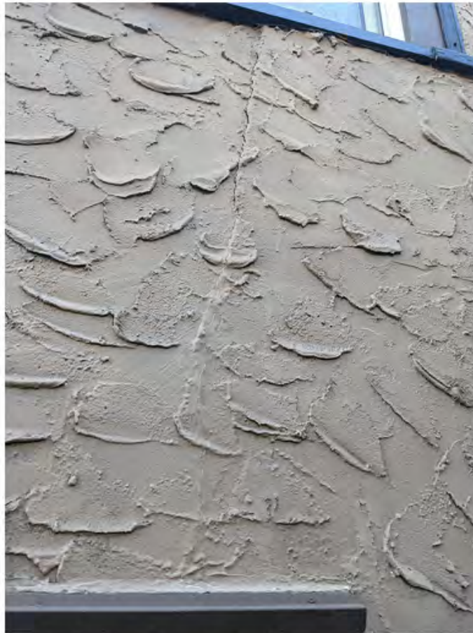
recently opened crack in stucco on east wall above crawl space access door.jpg
