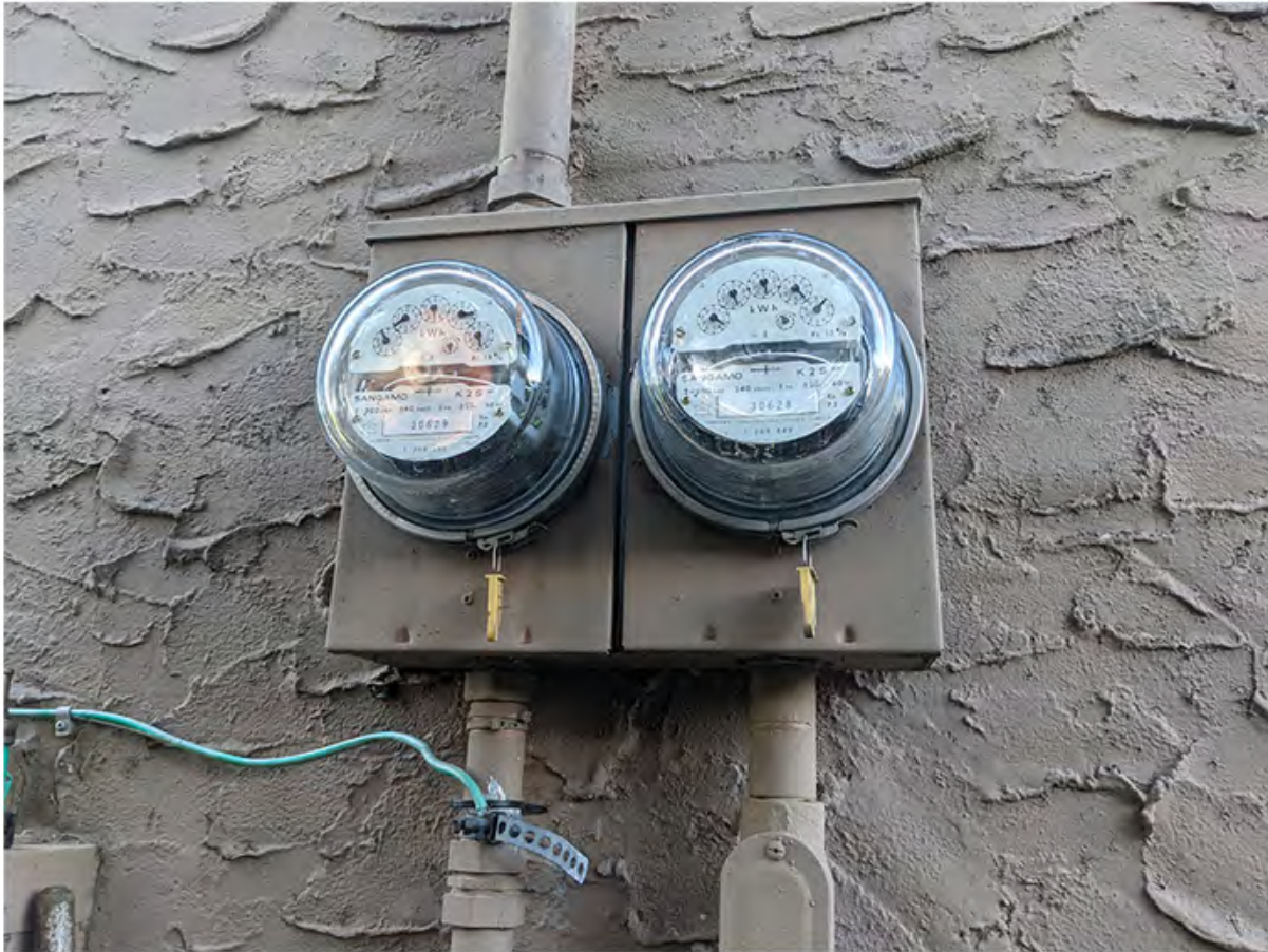
single phase electrical meters for both units on central east wall.jpg
