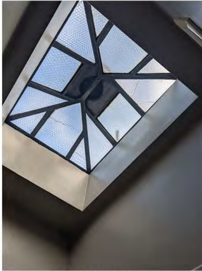
unit 351 - skylight with cracking.jpg
