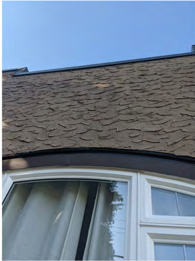
unit 349 - cracks in stucco above window.jpg
