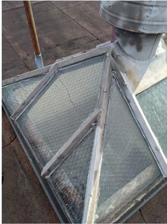
recent crack in skylight above unit 351.jpg
