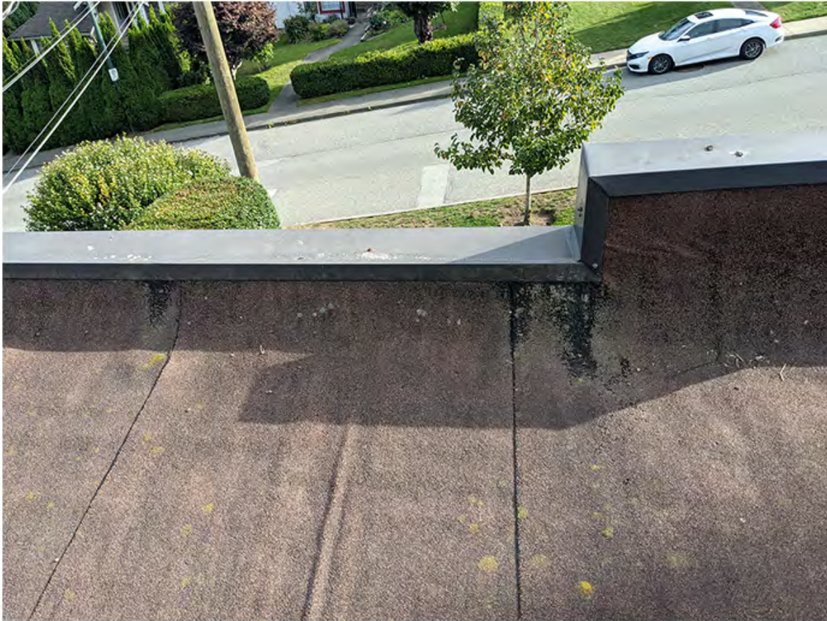
degraded granular material on south parapet.jpg
