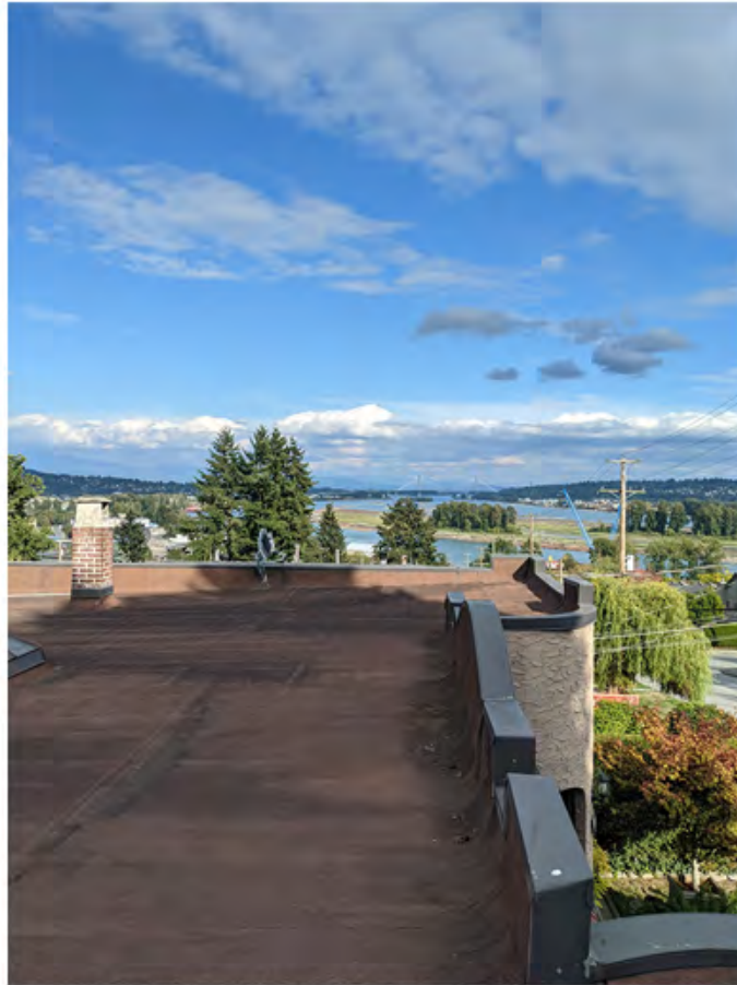
view of degraded rolled asphalt surface looking east.jpg
