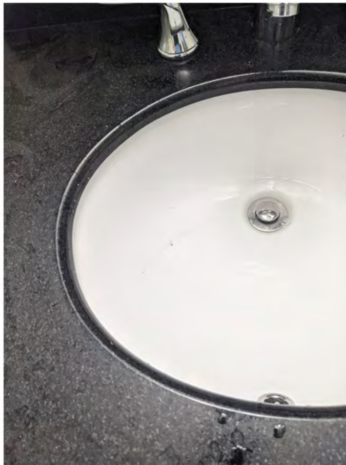
unit 349 - lower level bathroom sink needs replacement.jpg
