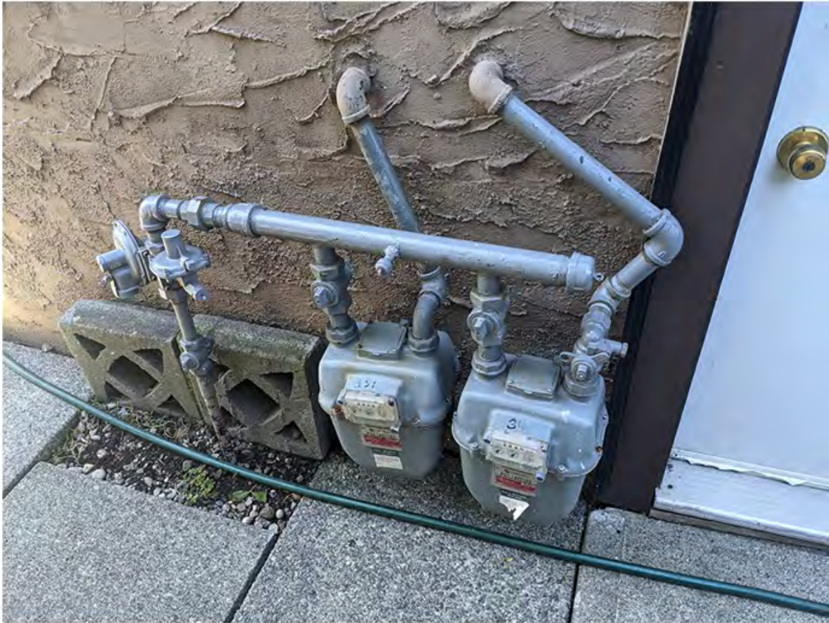
natural gas meters just south of crawl space access door on east wall.jpg
