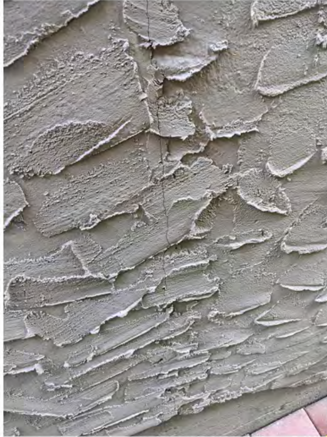
crack in stucco on west wall north side.jpg
