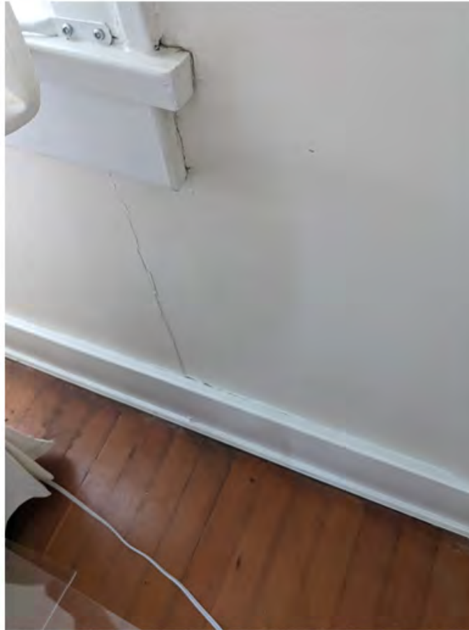
unit 351 - evidence of foundation settlement on south wall below window on main level.jpg
