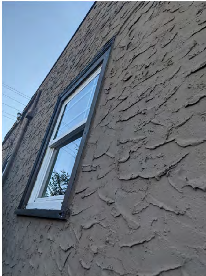
unit 349 - east wall window with no drip guard flashing above or below.jpg
