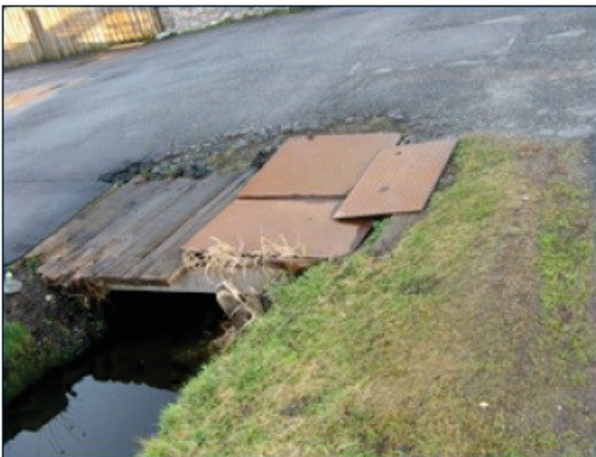
Existing non—standard rotten wood retaining wall
