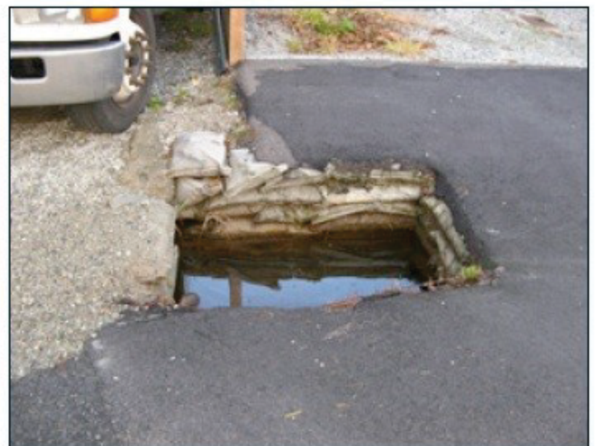
Existing hazardous gap between two driveway culverts
