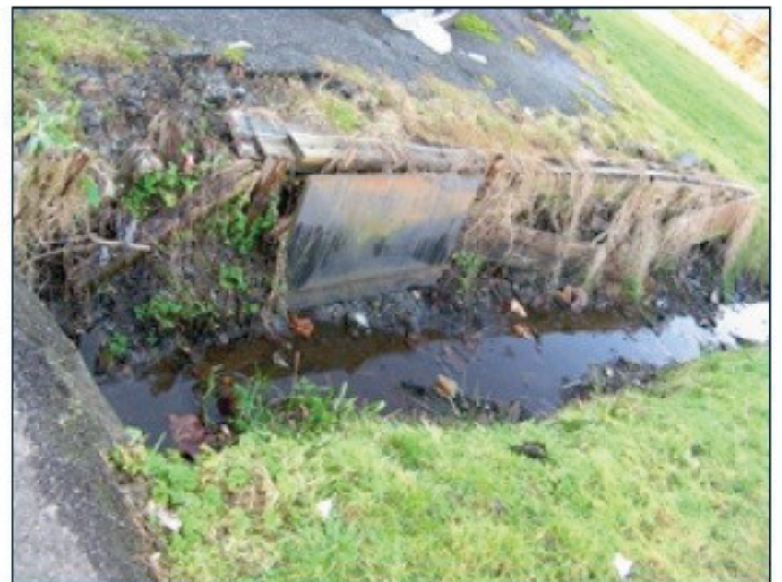
Existing hazardous pedestrian ditch crossing
