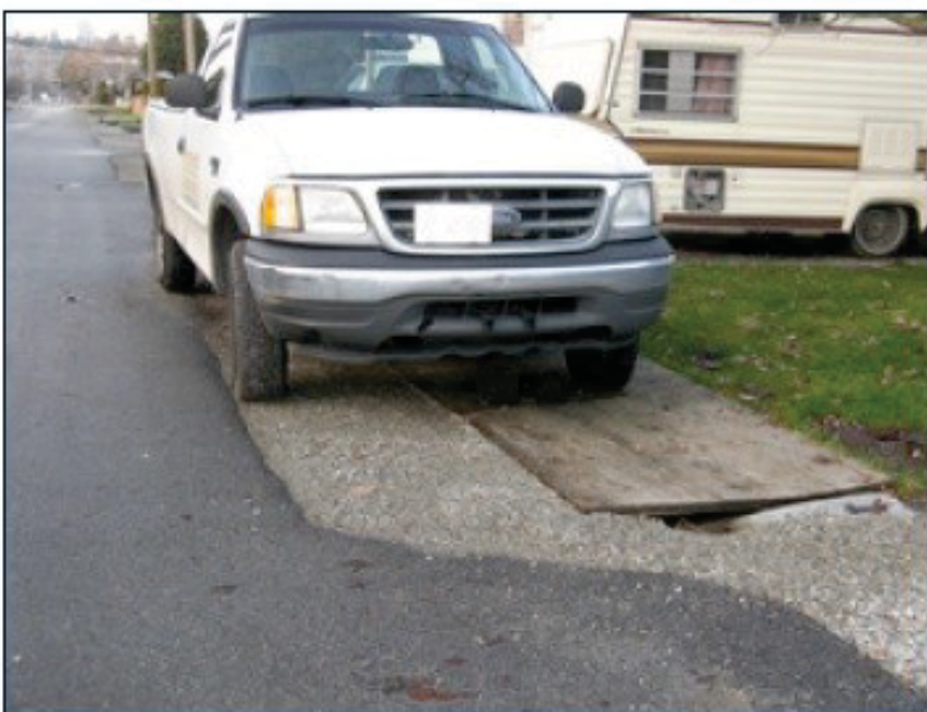
Existing hazardous plywood ditch cover
