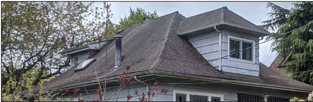
Fig. 21: Front view of the roof of Calbicks House at 208 Fifth Avenue, 2019, with the taller chimney visible in the foreground and the smaller along the roof line. (Source: Cummer)
