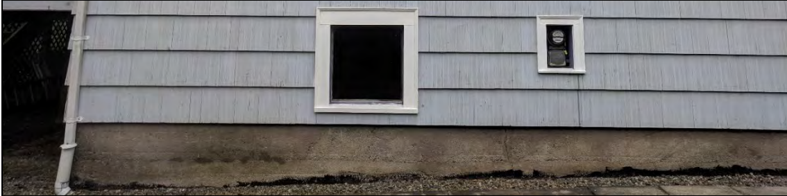
Fig. 18: Eastern side view of Calbicks House at 208 Fifth Avenue, 2019, illustrating its foundation. (Source: Cumber)
