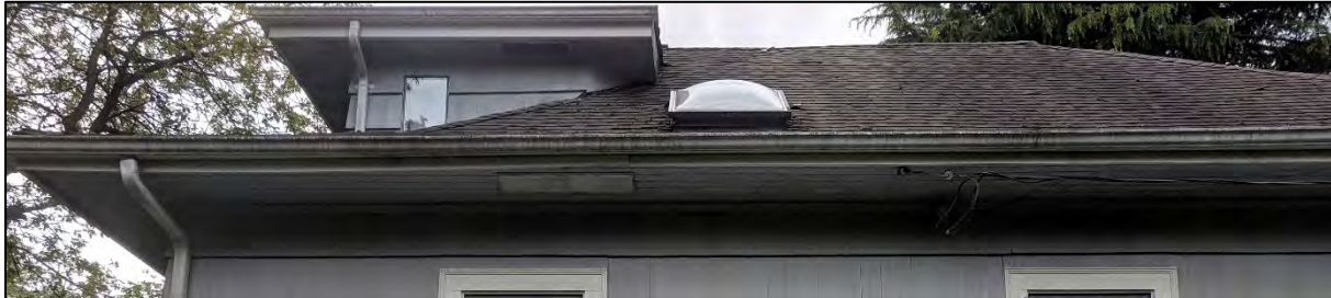
Fig. 20: Eastern side view of the roof of Calbicks House at 208 Fifth Avenue, 2019, with the unsympathetic skylight visible in the middle. (Source: Cummer)
