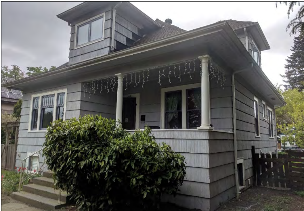
Fig. 19: Northwestern front and side view of Calbicks House at 208 Fifth Avenue, 2019, illustrating the overall good condition of its exterior wood elements. Note the landscaping possibly growing too close to the foundations, as discussed in section 9.9 below. (Source: Cumber)
