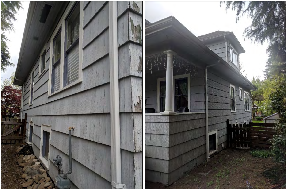
Figs. 11 and 12: Western side view of Calbicks House at 208 Fifth Avenue, 2019, from the back (left, Fig. 11) and the front (right, Fig. 12). Note the double-hung horned wood windows and the square wood windows. (Sources: Cummer)
