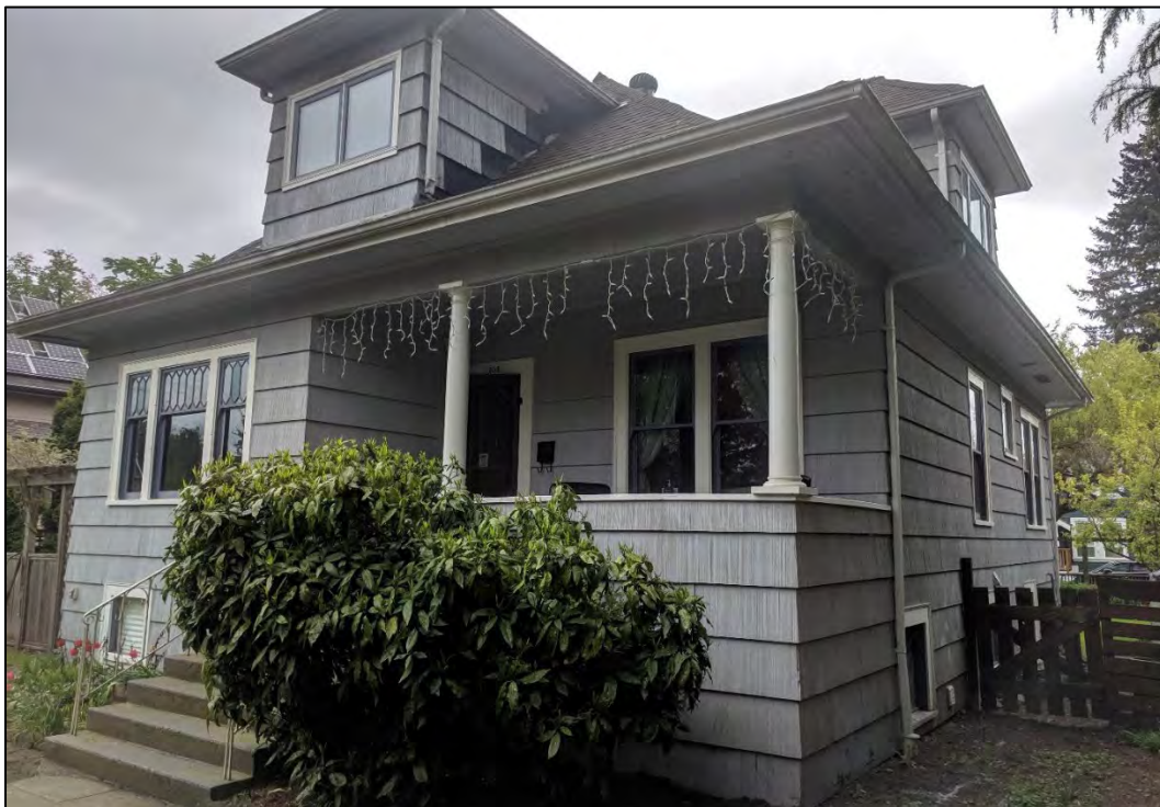
Fig. 19: Northwestern front and side view of Calbicks House at 208 Fifth Avenue, 2019, illustrating the overall good condition of its exterior wood elements. Note the landscaping possibly growing too close to the foundations, as discussed in section 9.9 below. (Source: Cumber)
