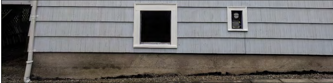
Fig. 18: Eastern side view of Calbicks House at 208 Fifth Avenue, 2019, illustrating its foundation. (Source: Cumber)
