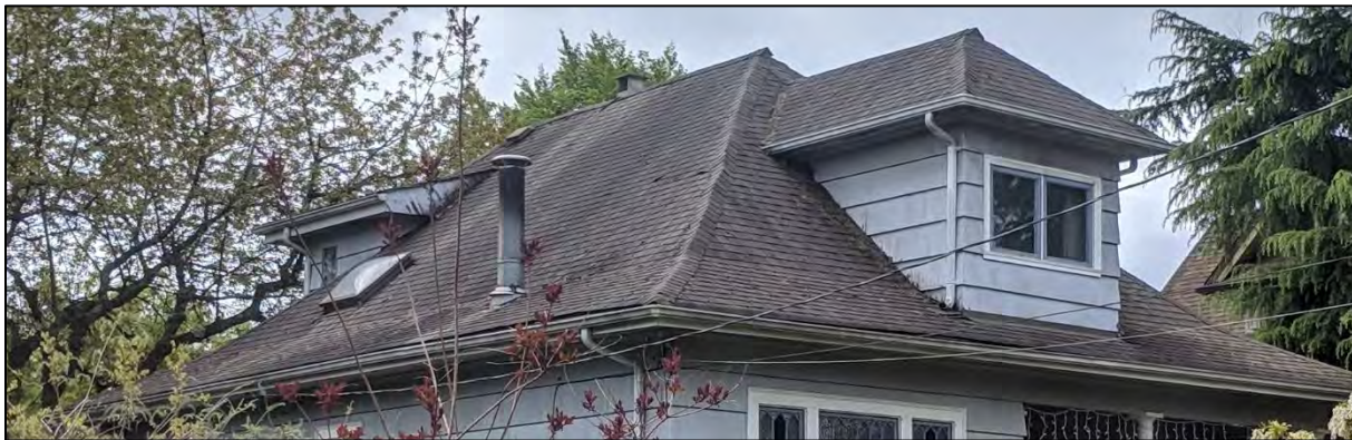
Fig. 21: Front view of the roof of Calbicks House at 208 Fifth Avenue, 2019, with the taller chimney visible in the foreground and the smaller along the roof line. (Source: Cummer)
