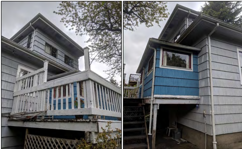
Figs. 16 and 17: Fig. 16 (left) shows the southwestern back view of Calbicks House at 208 Fifth Avenue, 2019, and Fig. 17 (right) shows the southeastern back view, illustrating some of the deterioration. (Sources: Cummer)
