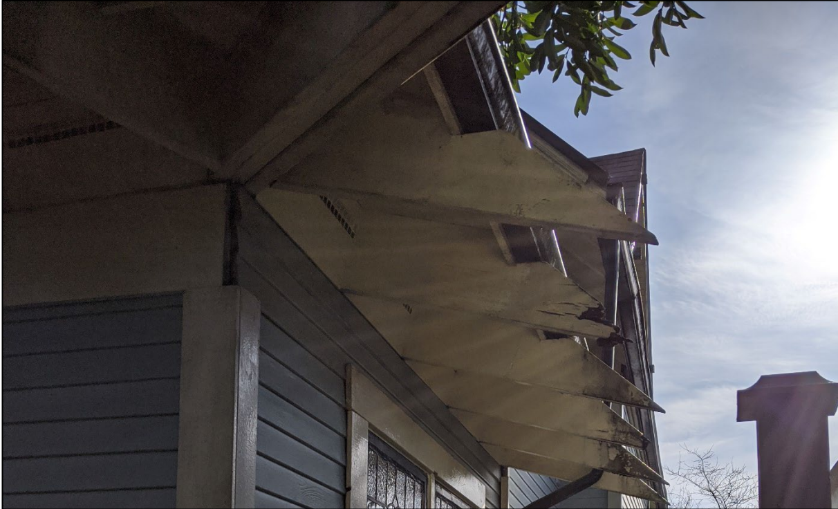
Fig. 12: Western side of Adams House at 515 St George Street, showing the dirty rafter tails, in need of cleaning and repainting, as well as ones in need of repair. (Source: Cummer)
