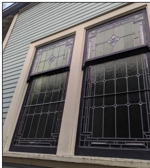
Fig. 16: Illustration of some of the original windows of Adams House, in this case a pair of double-hung horned wood stained-glass windows, showing a dirty sill that can be easily addressed. (Source: Marino)
